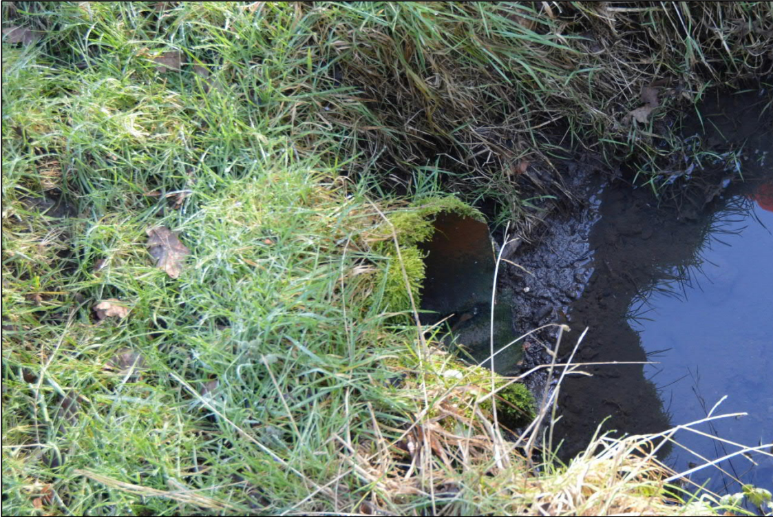
Photograph 3: Existing overflow pipe into the Bushburn Brook, within area of proposed, looking south-east
