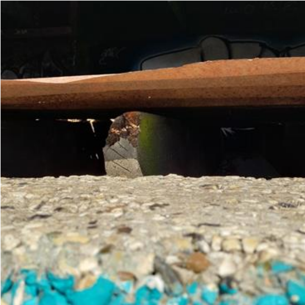
Figure 4.15: First-floor door opening depicting the joists sitting above the sill of the doorway
