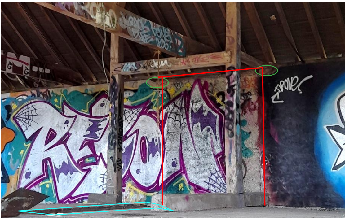
Figure 4.10: View of the ramp and H-framed timber structure from the first floor. The ramp is situated in the gap in the floor, outlined in blue. The original location of the lintel ends are circled in green and the red lines depict the location of the former opening.
