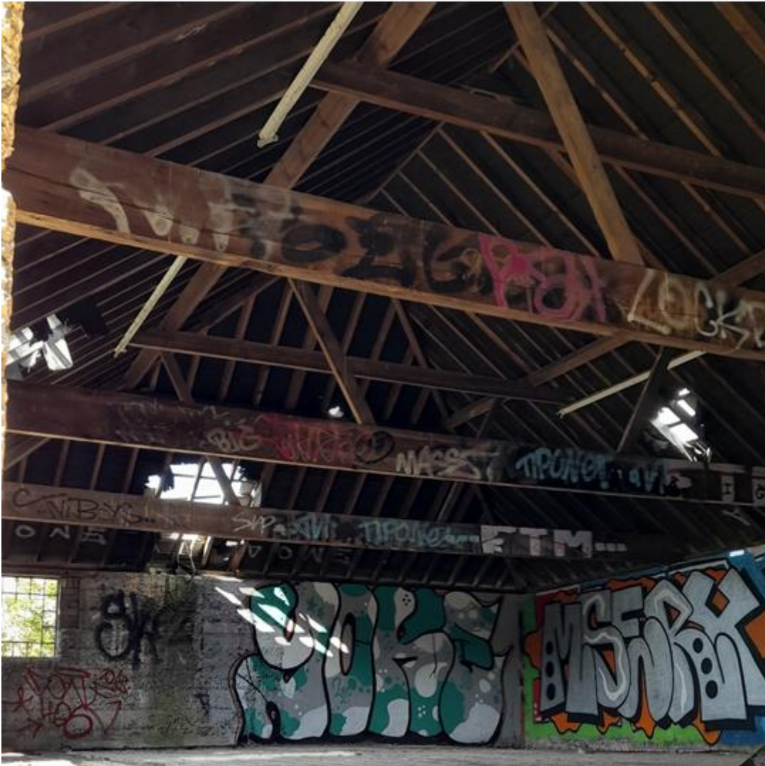
Figure 4.16: First floor of the Concrete Barn showing the timber roof trusses, holes in the roof and the strip lighting (outlined in blue).
