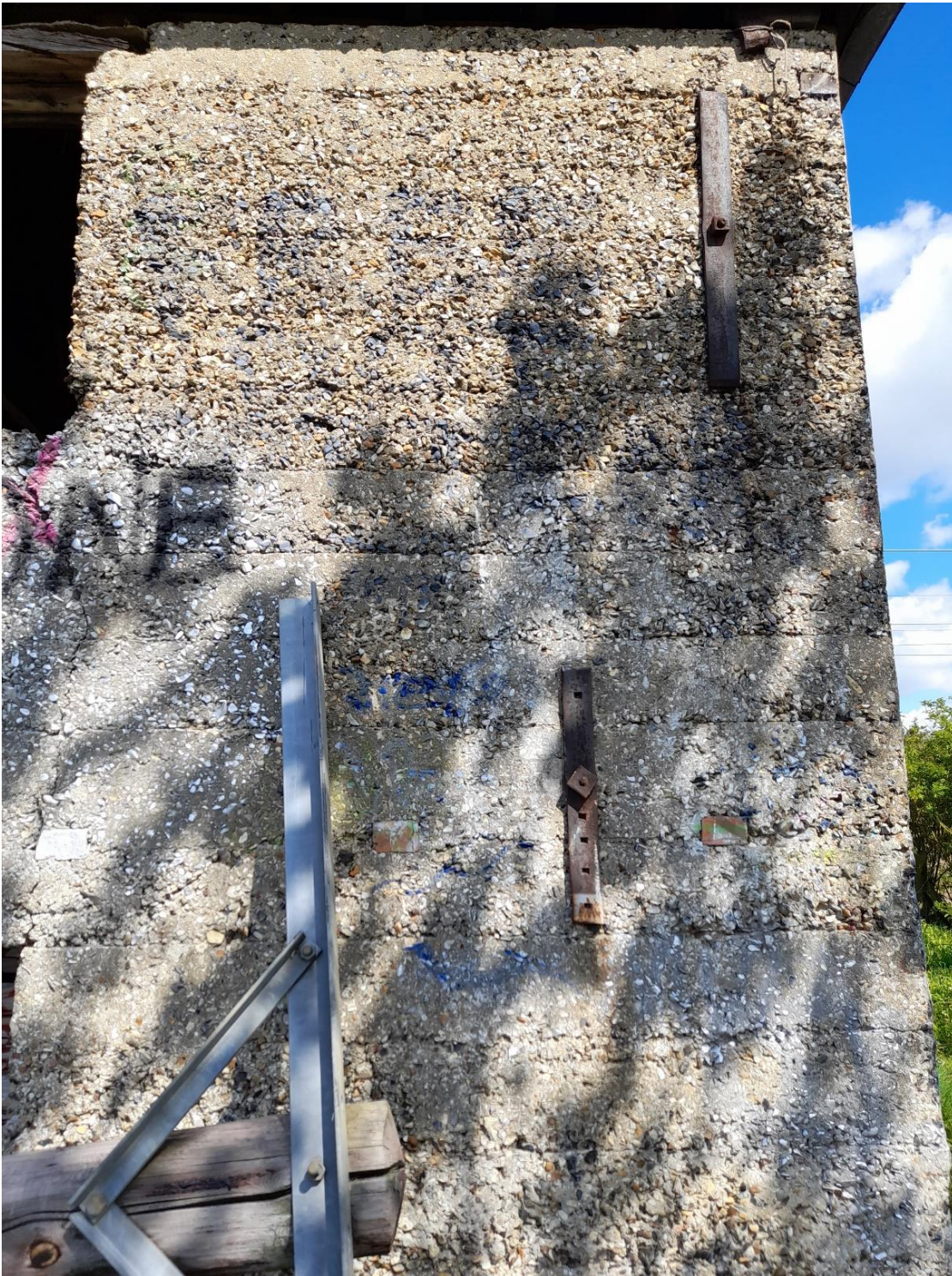
Figure 5.1: Eastern corner of the southern elevation, depicting the stripes left from each pour of the concrete.
