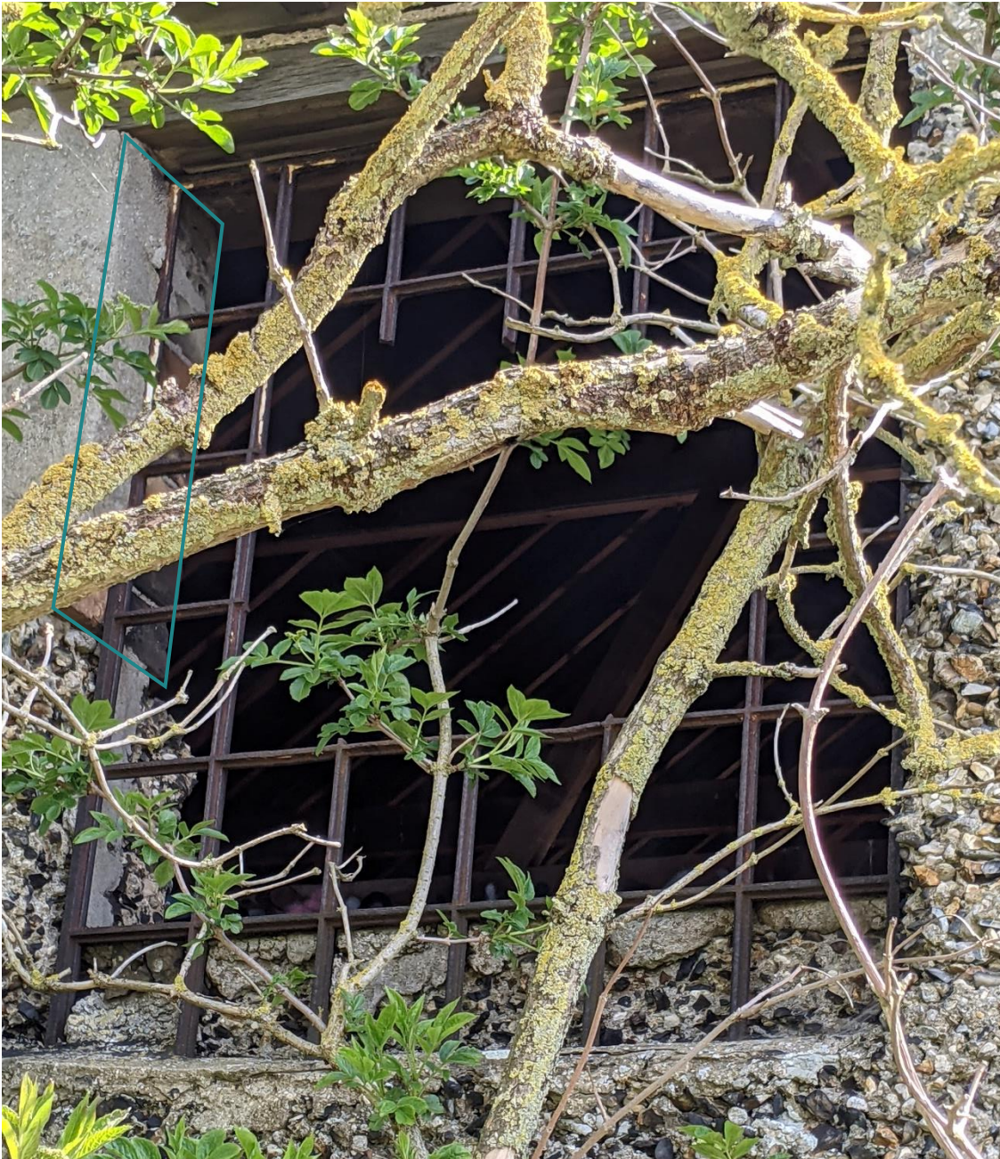
Figure 4.12: The best example of the cast iron windows of the Concrete Barn, on the western elevation. There is evidence of later brick infill to the upper left of the window, outlined in blue.
