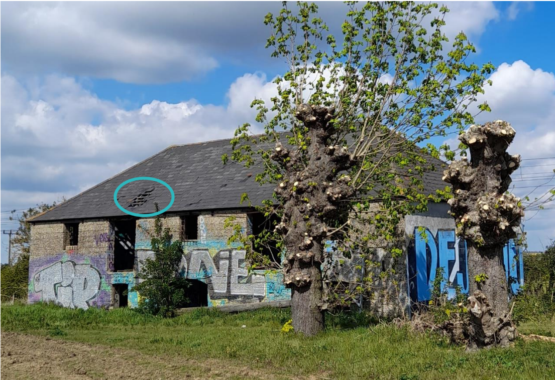
Figure 4.17: Exterior of the Concrete Barn showing the relatively new roof tiles and area of missing tiles circled.
