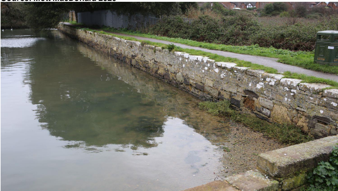
Figure 4.9: View of scheme area looking South showing previous sea defence wall. Source: Mott MacDonald 2020
