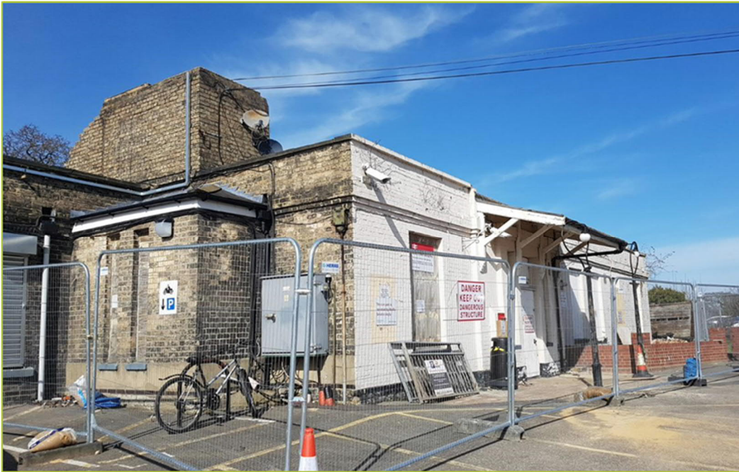
Figure 2: Saxmundham station today, after underuse, fire and first-floor demolition.
