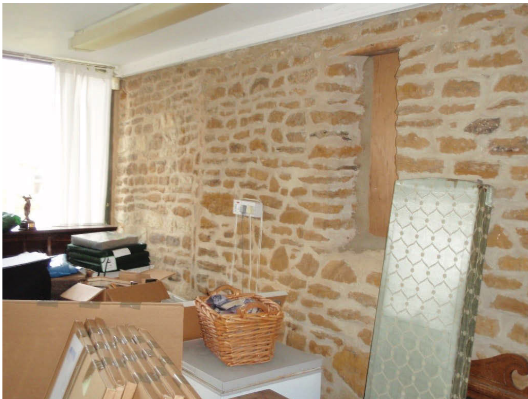
Plate 14: Games room showing stonework jointing and blocked ventilation slit in NE wall
