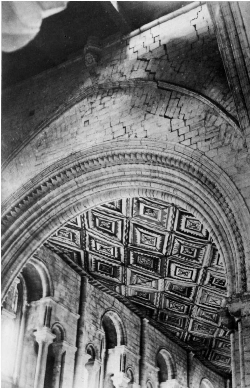
Figure 4. Pre-1880s photograph showing a section of the North Transept Ceiling as well as significant structural cracks in the north crossing arch wall. 9 Evidence suggests the ceiling painted decoration is significantly different from the thirteenth-century linear design. It is probable the alterations were made in the 1740s and that scheme was simply repainted in the 1830s.
