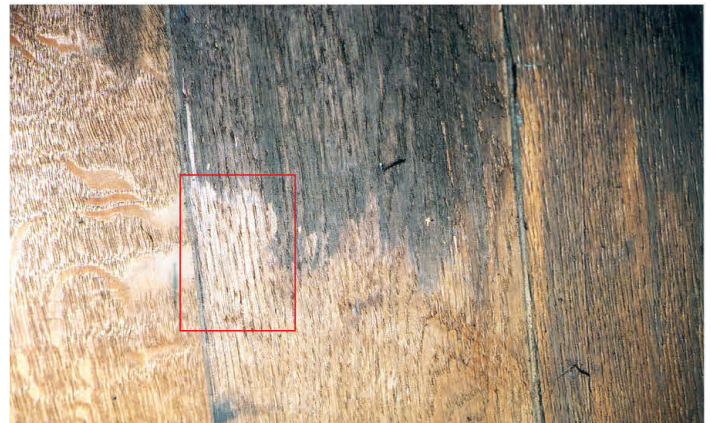
Plate 4. Detail of an area of the darkened coating, following soot and dirt removal, from which samples were obtained for analysis (Sample 1). The red square shows the location of a small test to remove the coating with IMS. The underlying wood surface is marginally lighter than the uncoated surface.
