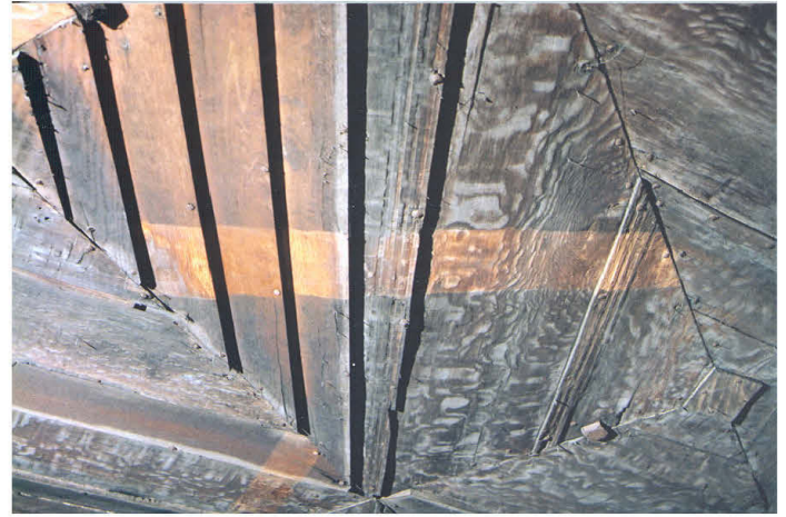
A surface cleaning test using wishab sponges to remove the thick accretions of soot and surface dirt across original and 1890s ceiling boards.
