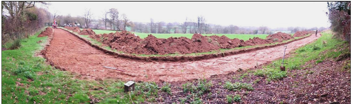
Figure 32. Panorama photograph of the last stage of the excavation for the new access road. Viewed from the northern corner of the field under excavation. Looking south, downslope. The Former Operations Block is in the left – background. 1m scale within the trench.
