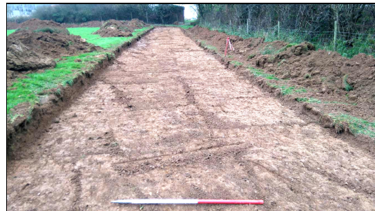
Figure 34. The eastern arm of the watching brief trench. Surface of geology 103 exposed. Looking WNW from 331630 / 107370. 1m scale
