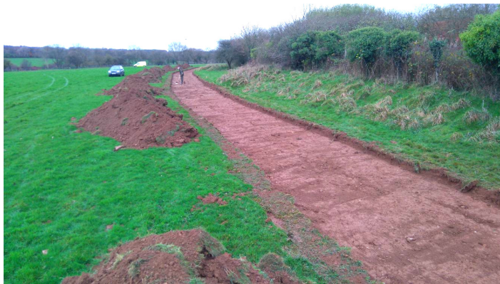
Figure 29. The northern arm of the watching brief trench. Base of subsoil 102 / surface of 103 exposed. WWII landscaping banks. Looking WSW from 331550 / 107350.
