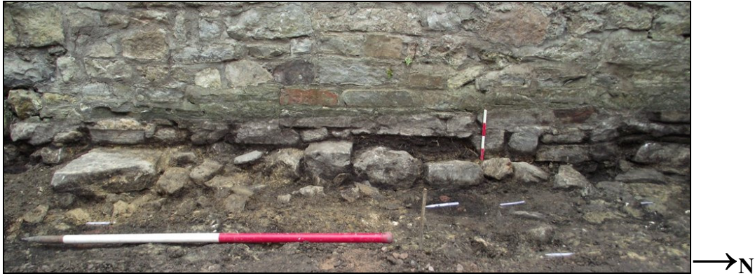
Figure 33 – Off-set foundations (261) butting up to retained masonry (264). The vertical scar line between walls (280) and (279) is visible on the left side of the photograph.
