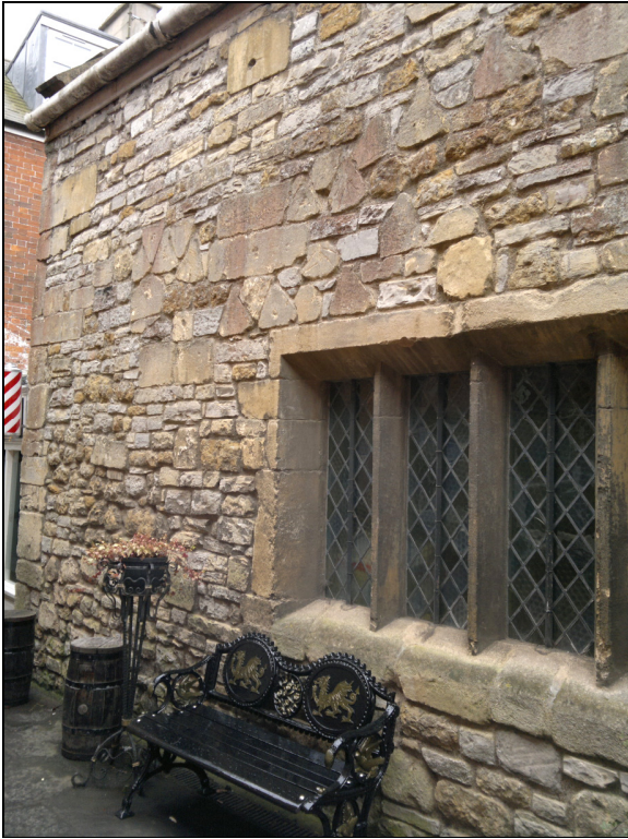
Figure 40. The distribution of re-used yellow freestone ashlar and moulded stone in the east face suggests that Room 4 may have been built in two or three phases. The lower courses contain few blocks of re-used stone, the window and much of the upper courses appear to have come from Glastonbury Abbey, and the upper-most courses are made of Lias block which are much less worn than those in the lower courses.
