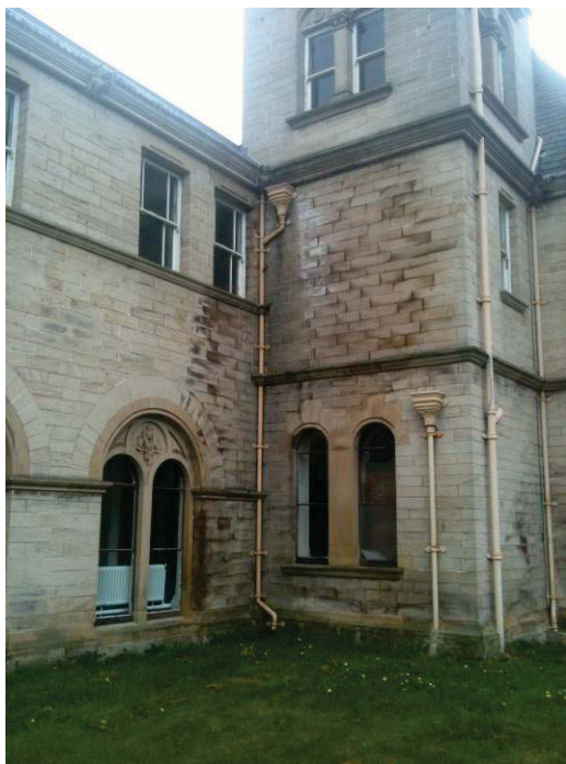
Figure 37 South façade, angle between central tower and 1870s former chapel corridor showing water-damaged masonry. This damage is caused by inadequate 1870s rainwater goods, and there is evidence of dry rot fruiting bodies internally.
