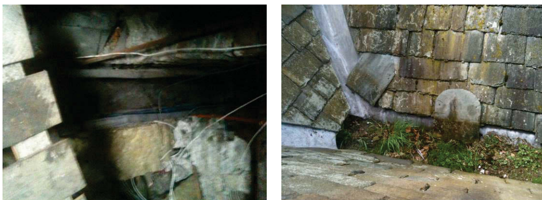
Figure 34 The lead-lined internal channel on the left, with the valley on the right, showing it blocked with debris, weeds and slipped slates.
