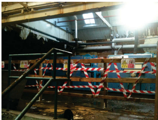
Figure 75 Interiors in poor condition with former laundry machinery.
