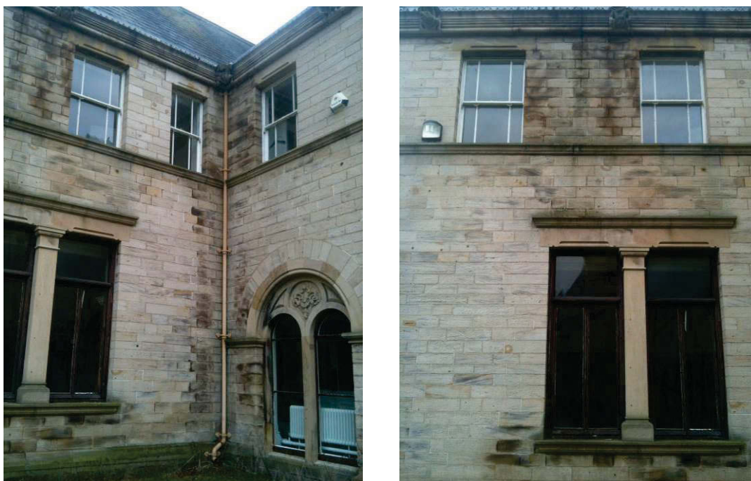
Figure 40 South façade, angle between former billiards room and 1870s former chapel corridor showing water-damaged masonry.
