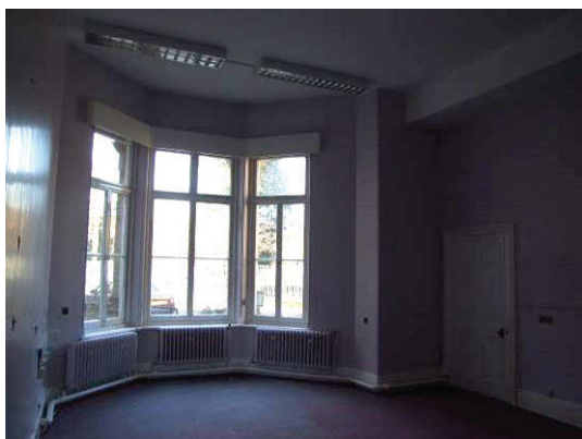
Figure 62 Room with bay window and load-bearing beam above right. This may be where the c.1870 hall end wall was, and this room may have been an external courtyard.
