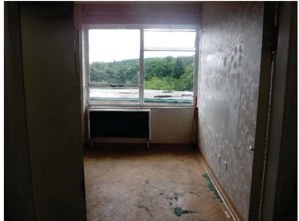
Plate 141 Building 31, McCoull Clinic interior, first floor office with blocked communication hatch. Facing south-east [1898]
