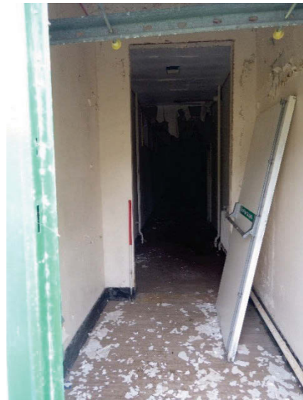
Plate 71 Building 18 Tredgold Hall, interior circulation corridor with removed partition walls. Facing south. [3015]
