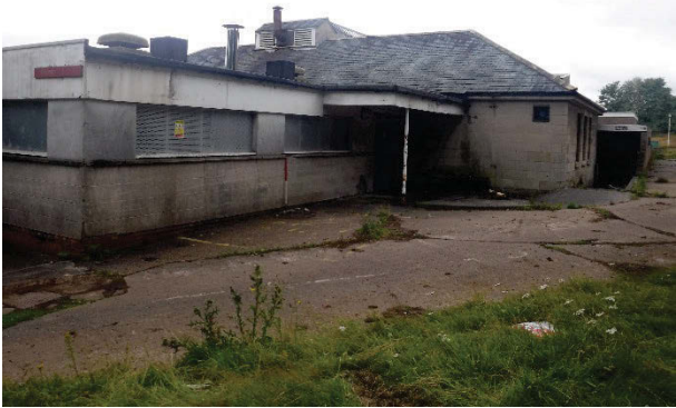
Plate 150 Building 34, Derwent Kitchens and Dining Hall exterior, rear elevation with north-east annexe. Facing south [2546]
