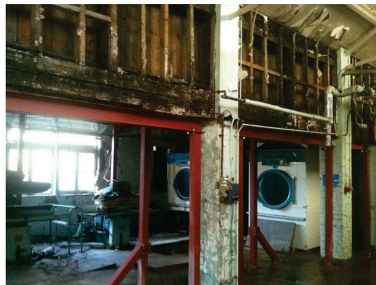
Figure 76 Looking south, under propped timber lintols, into the former carriage shed. Laundry machinery beyond.
