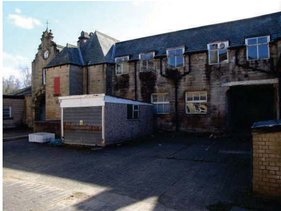
Figure 73 The 1870s stable range, altered several times, with the 1889 enclosed bridge to the church, relocated on the left, and a 1970s garage in front. The dormer windows have been inserted with little consideration for rainwater shedding.
