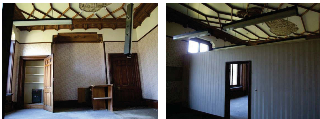
Figure 57 Dining room, with buffet-table recess on the left and partition on the right. The fallen area of the plaster ceiling is clear.
