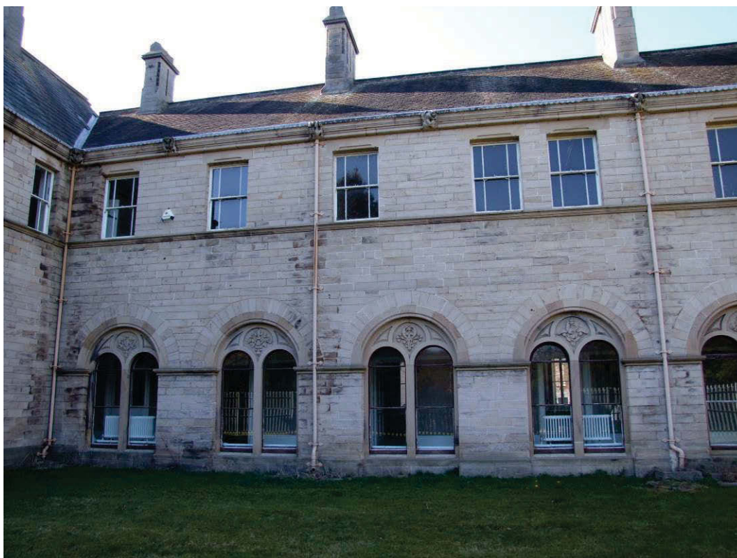
Figure 39 South elevation to terrace garden, showing leaking downpipes, and damage at west angle.
