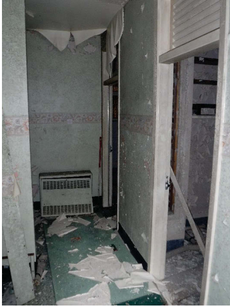
Plate 265 Building 69, Darwin & Seguin, internal corridor, west end south pavilion wing. Facing west. [2562]
