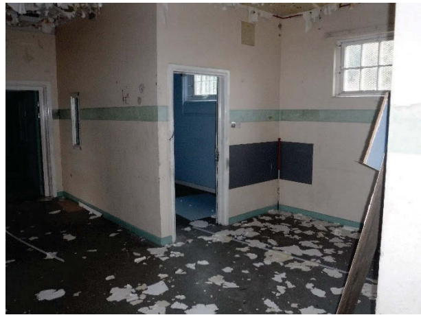
Plate 62 Building 17 Brinkburn ground floor internal hallway with partitioned former cloaks and boots room [1692]
