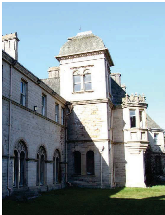
Figure 36 Central tower which has lost its brattishing.
