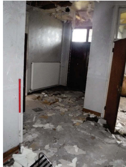
Plate 197 Building 40, Alison interior central wing main internal corridor with exterior doors. Facing east. [2185]
