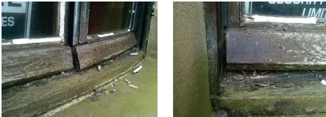
Figure 42 Ground storey casement window showing failing cills.
