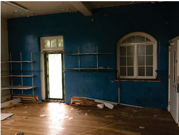
Plate 89 Building 24, Tyne Villa interior, east wing southern partitioned dining room. Facing west. [3090]
