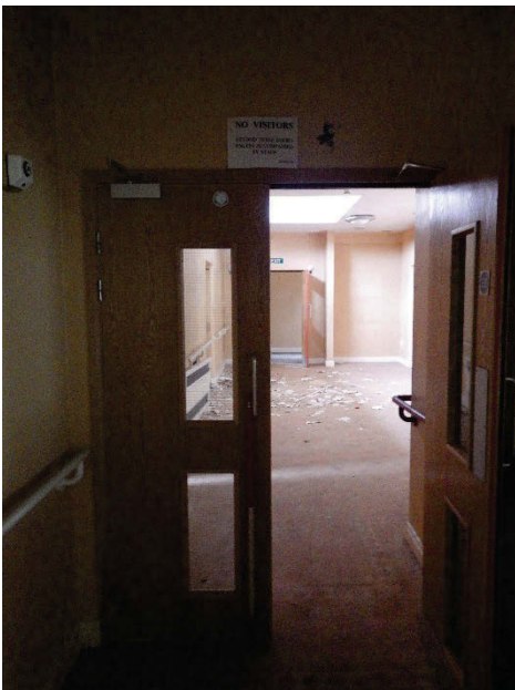
Plate 46 Building 13 Midway/Janie Hepple Unit interior corridor and hallway with restricted access. Facing north-east [1591]
