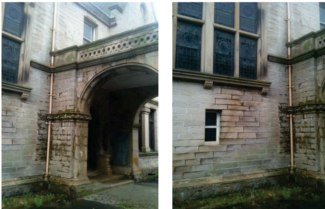
Figure 41 Ground storey, north entrance façade, porte-cochère , showing water-damaged masonry and slipping voussoirs.
