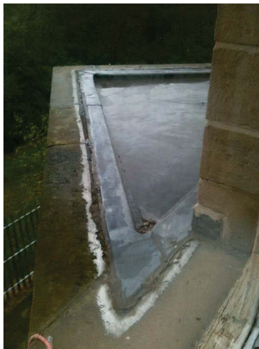
Figure 38 Roof to the south-west square bay-window. It is a poor piece of leadwork and is damaged. There is water damage internally.
