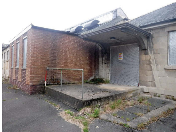
Plate 149 Building 34, Derwent Kitchens and Dining Hall exterior, south-east elevation and store-room access with porch. Facing north-west [2539]
