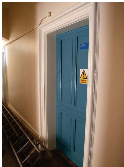
Figure 67 Former service wing ground storey corridor, showing old door and frame joinery.
