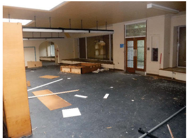
Plate 211 Building 44, Patients' Shopping Centre, general view room g24, 'shop female'. Facing north-east. [2138]
