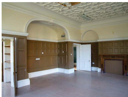
Figure 64 Billiards room looking towards the settee niche, and the blocked chimney piece. The original finish of the ceiling can be seen at the top of the image.
