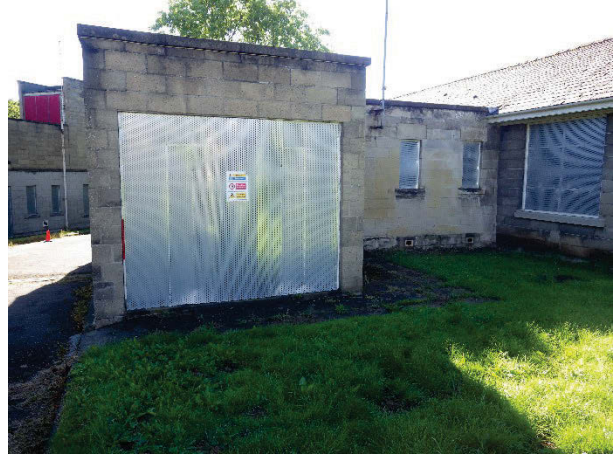
Plate 119 Building 30, The Close, exterior north (rear) elevation with north wing. Facing west. [1752]
