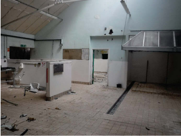
Plate 156 Building 34, Derwent Kitchens and Dining Hall interior, "main kitchen", subdivided. Facing north-east. [2492]
