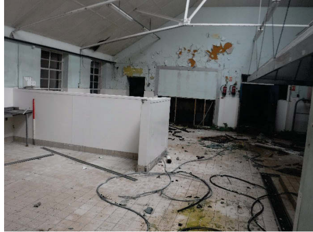
Plate 157 Building 34, Derwent Kitchens and Dining Hall interior, "main kitchen", subdivided; oven in background. Facing north. [2501]
