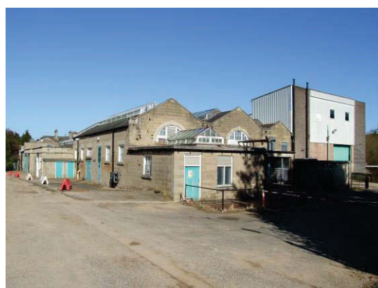
Figure 7 The former hospital laundry, built in the early 1920s, from the west. They are built in poor-quality reconstituted stone and have not been well-maintained. To the right, is the former hospital power station.
