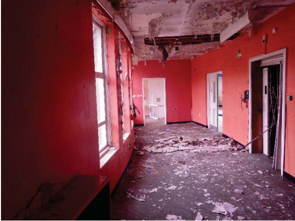
Plate 48 Building 13 Midway/Janie Hepple Unit curving corridor with lift shaft and blocking. Facing north [1613]
