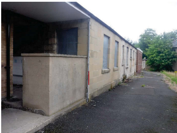
Plate 148 Building 34, Derwent Kitchens and Dining Hall exterior, south-east elevation and access. Facing north [2534]
