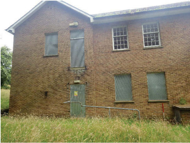
Plate 68 Building 18 Tredgold Hall exterior S gable end with removed external stair. Facing north. [3006]
