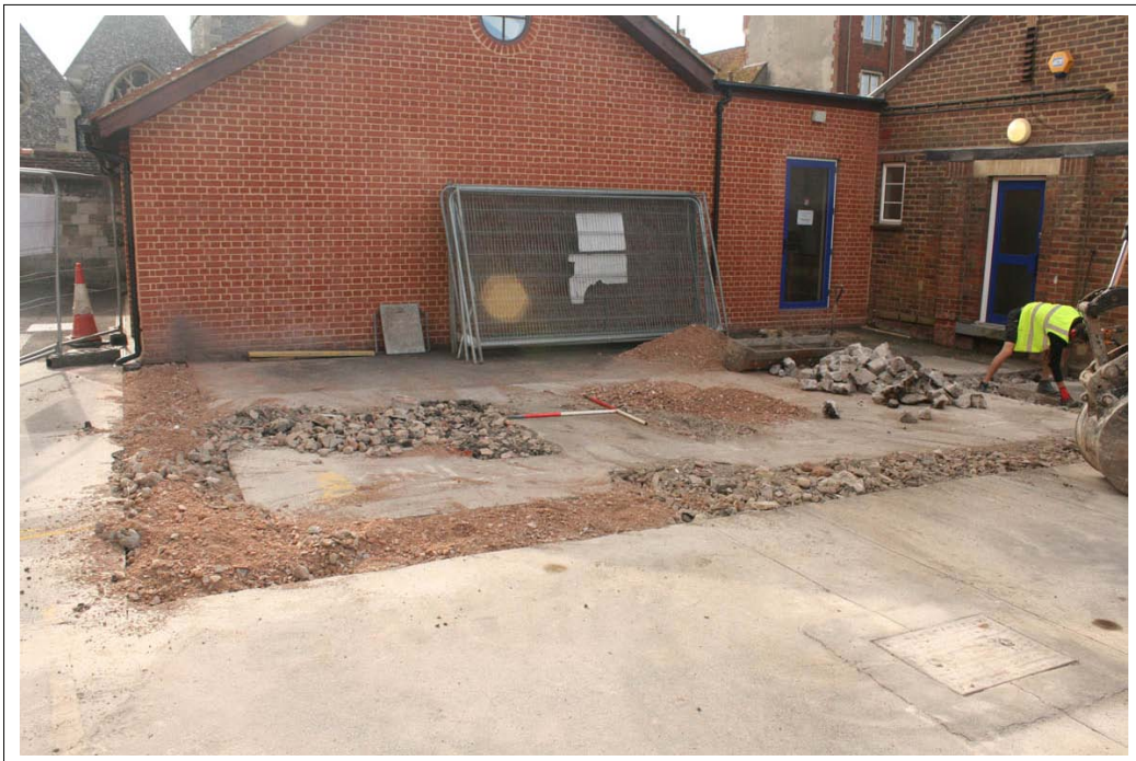
Plate 1: View of foundation trench layout after breaking up of concrete overburden. Looking east, scales 2x1 m
