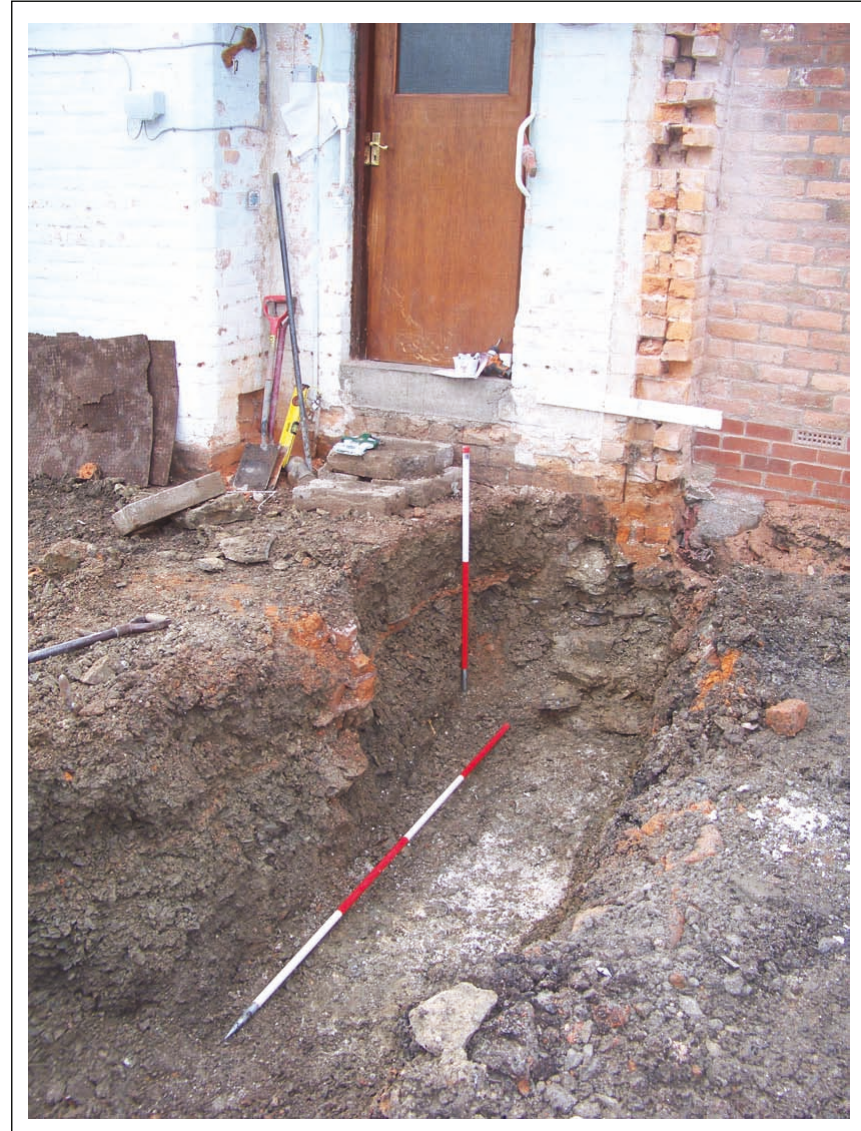
Plate 4 - Area B, with Mistress Yard Wall Footings and N. Facing Section. Looking SW. Note N S Brick Wall of Coal House in Section. Scale 1m x 2m.
