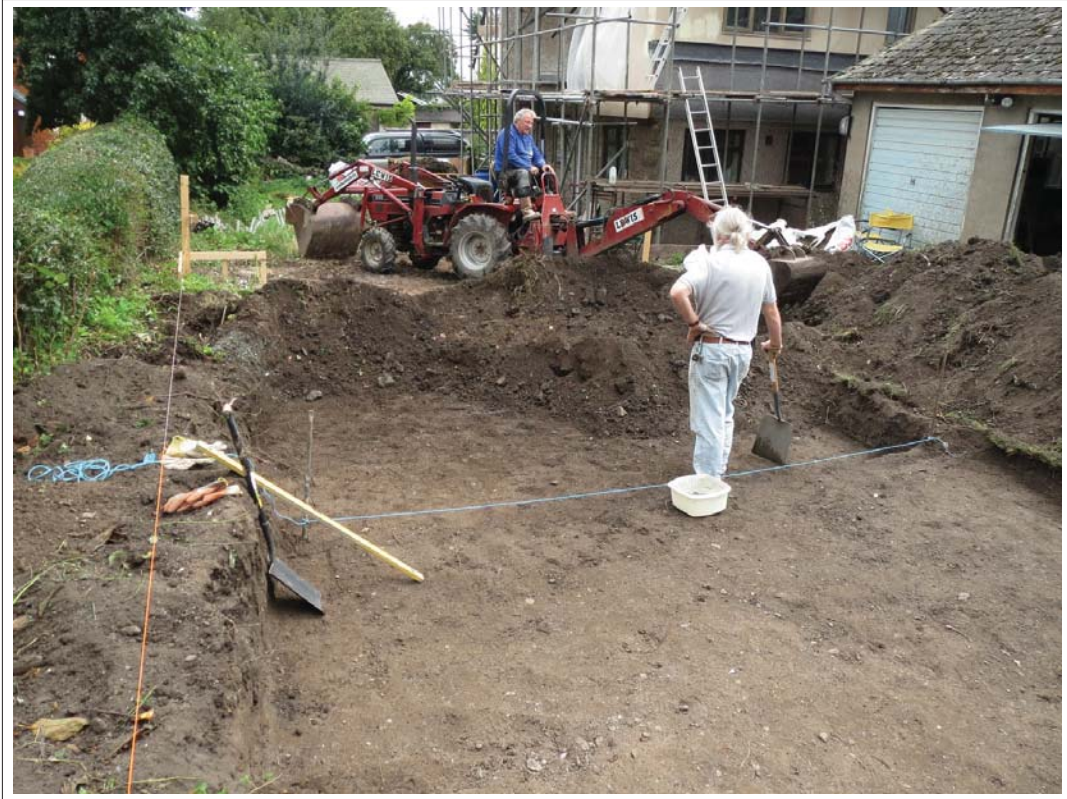
Plate 3. Area A: working shot of excavations for the garage foundations. Looking east-northeast.
