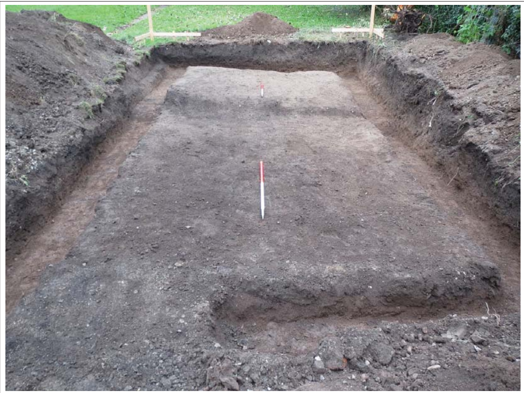
Plate 4. Area A: view of the reduced dig and footings for the garage. Scales: 2x1m. Looking west-southwest.
