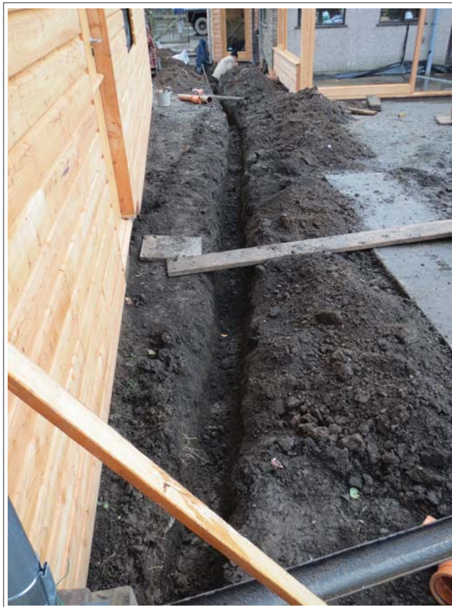
Plate 16. View of excavations for drainage extending along the new garage and sunroom. Looking east-northeast.
