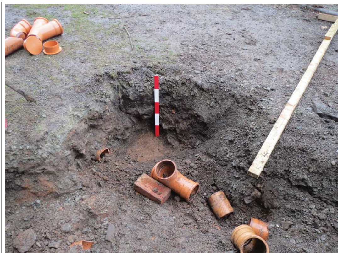
Plate 14. Excavations for drainage to the west of the porch, showing natural (302) below made ground (301) and driveway gravel (300). Scales: 1x0.5m. Looking northwest.
