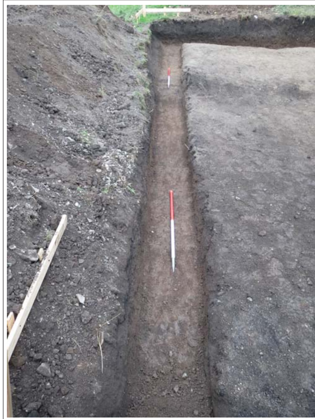
Plate 5. Area A: post-ex shot of the southern side of the of the garage foundations. Scales: 2x1m. Looking west-southwest.
