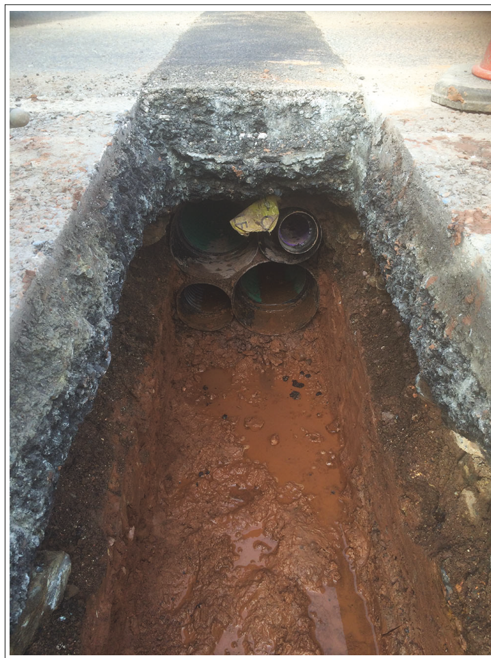
Plate 14. Shot of Cable Trench through road A454 taken during a Watching Brief in 2015. Looking south
