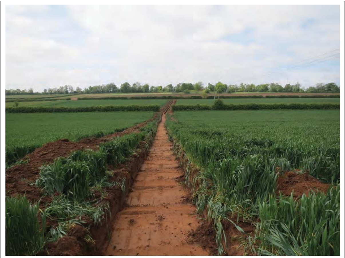
Plate 7: View along cable trench south west from crossing of A454 at Hermitage Farm in to Area 2
