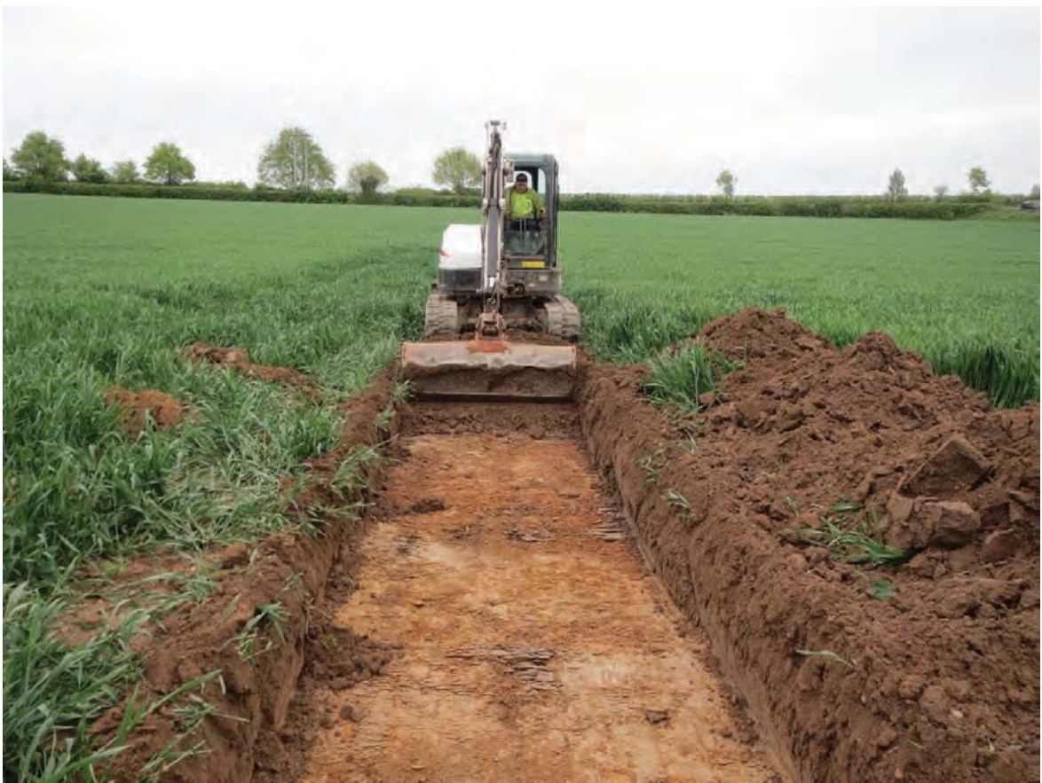
Plate 9: View of cable trench excavation, looking south east, between Area 1 and A454 road crossing at Hermitage Farm
