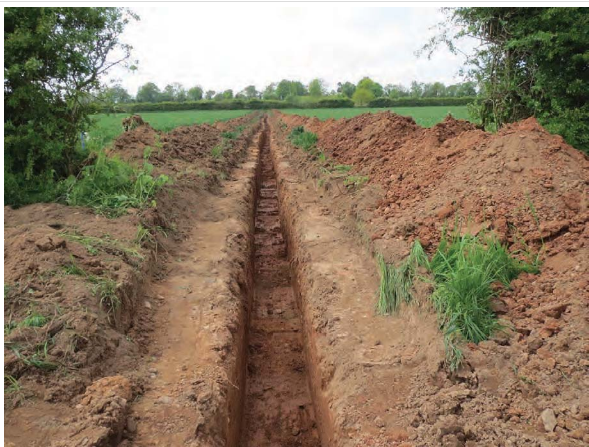
Plate 10: View of cable trench through field boundary at Area 2. Looking south west
