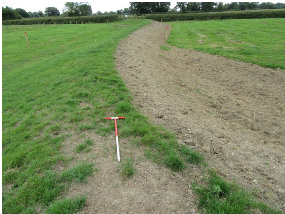
Plate 2. East facing view of flood embankment prior to main groundworks, 1m and 0.3m scales
