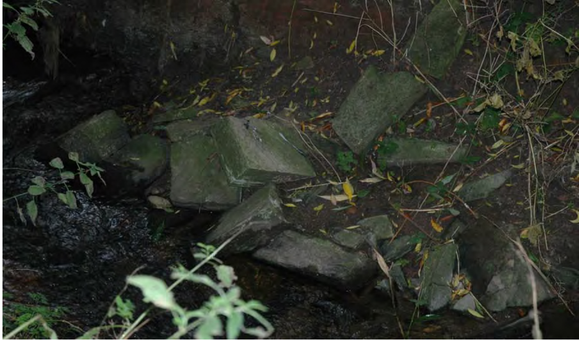
Plate 5: Collapsed stone lining to the ditch which runs along the western boundary of the site
