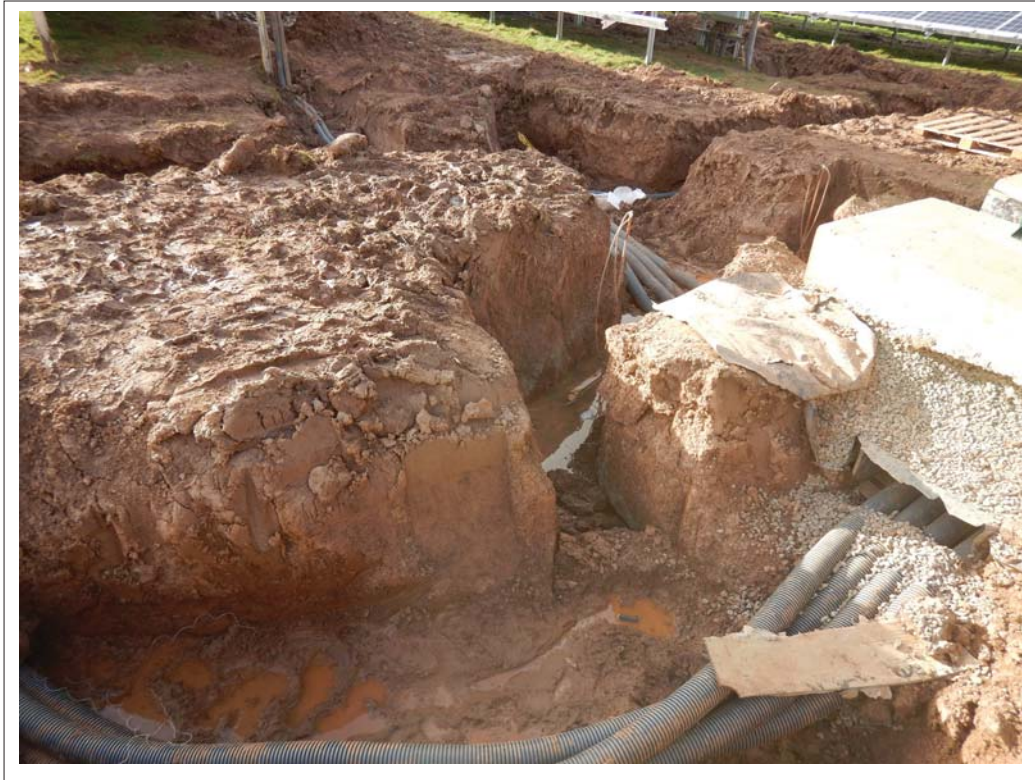
Plate 5. Close up of cable trenches within Field 1. Looking north-west
