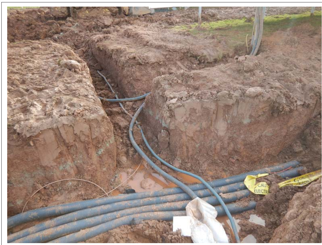
Plate 2. Close up of cable trenches within Field 1.
