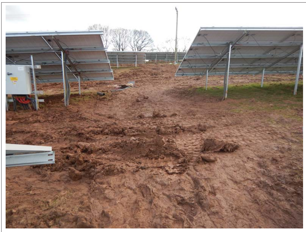
Plate13. General shot of backfilled cable trenches in central area of Field 2. Looking south
