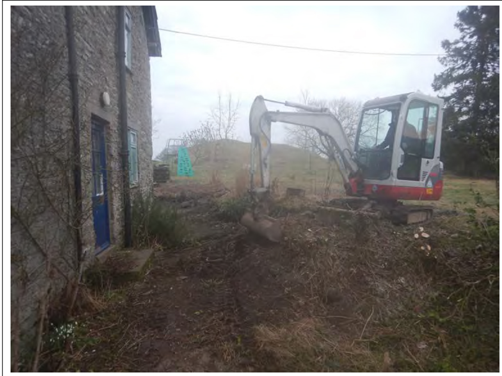
Plate 1. Removal of topsoil and subsoil prior to the excavation of evaluation trench (with Motte visible in background), looking north.
