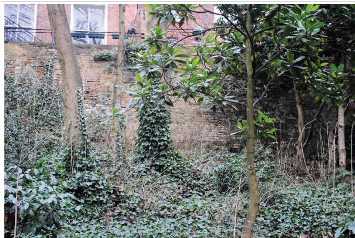
Plate 20. The retaining wall at the top of the escarpment, to the rear of the Old School House. Looking southeast.
