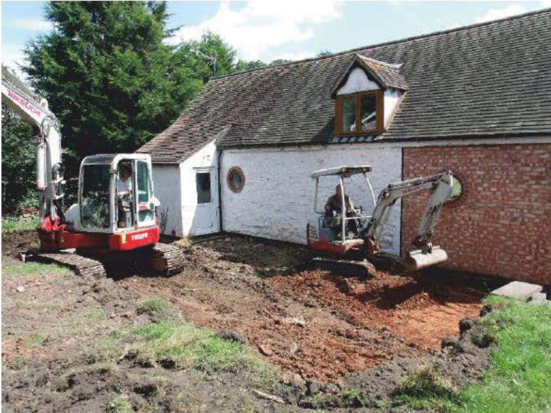
Plate 25: View of end of the works for Trench 2 at the rear of the house; shot facing E
