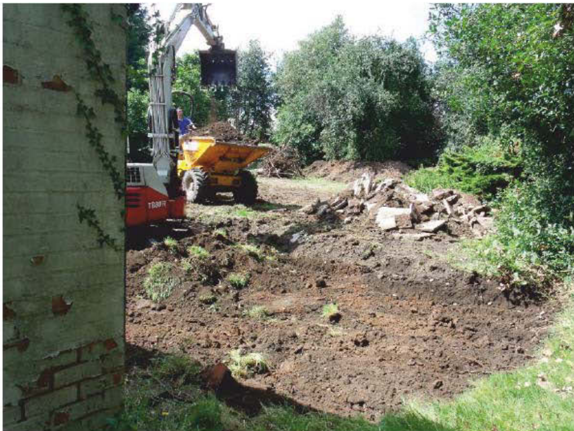
Plate 26: View of end of the works for Trench 2 at the rear of the house; shot facing W
