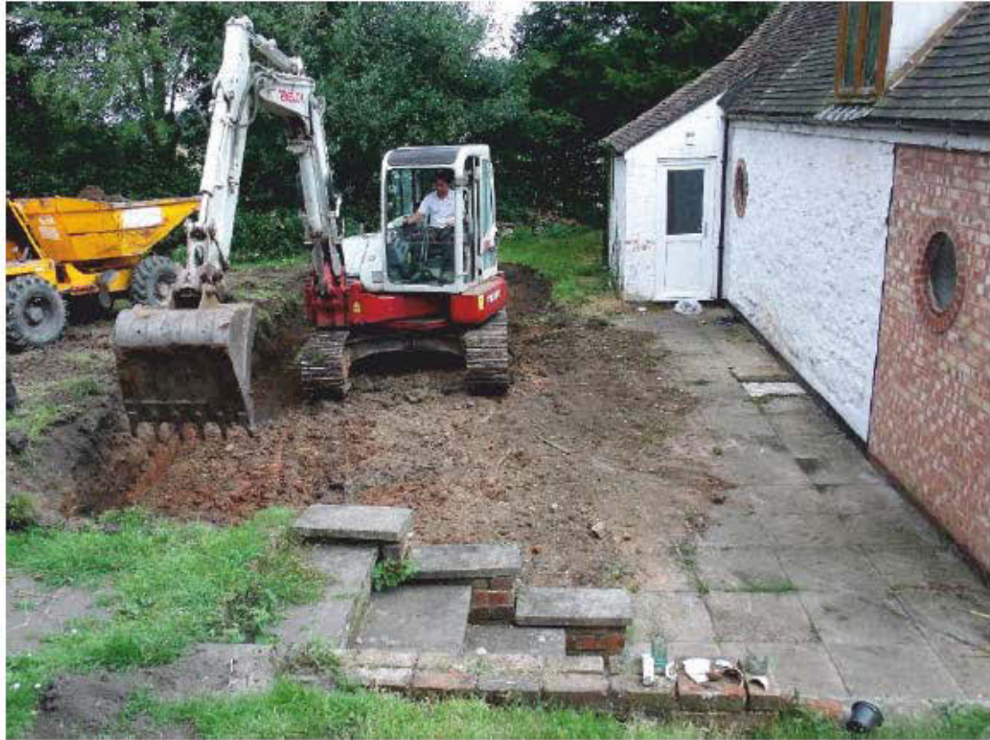
Plate 19: View of works for Trench 2 at the rear of the house; shot facing NE
