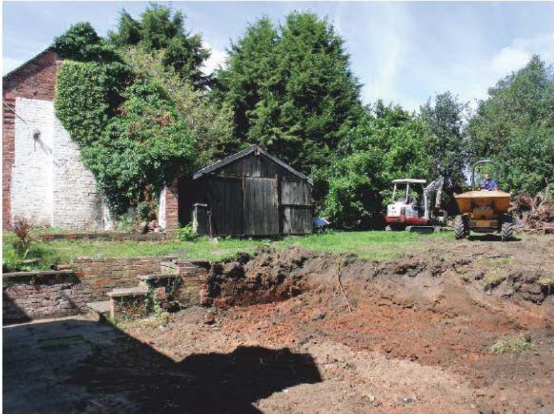
Plate 21: View of works for Trench 2 at the rear of the house; shot facing W
