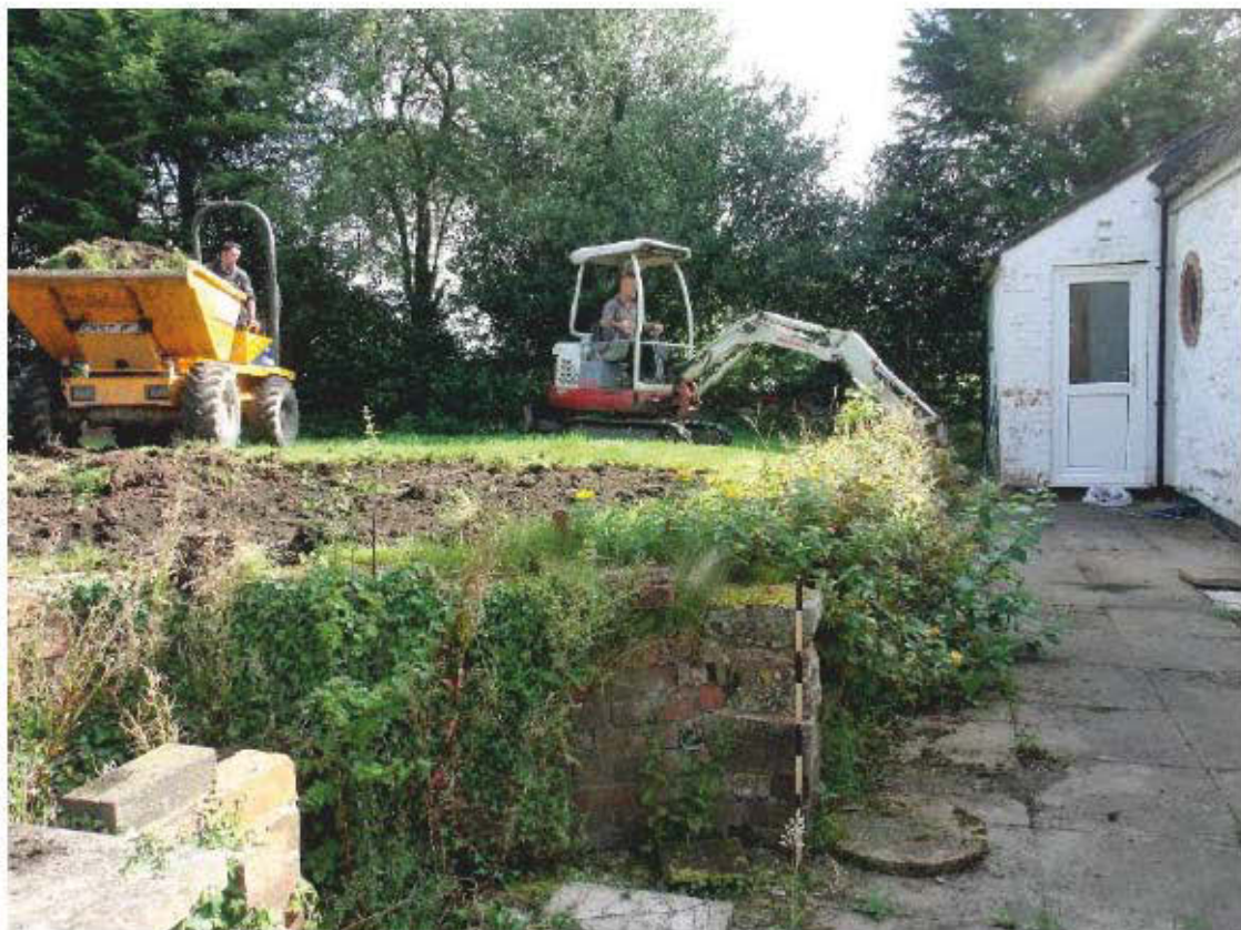
Plate 16: View of works for Trench 2, and brick garden wall [205] at the rear of the house; shot facing NE
