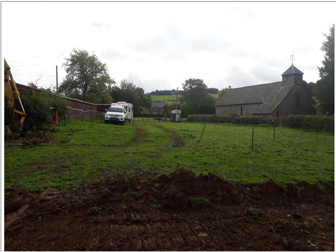
Plate 1. Eastern end of excavations. View E towards church, showing undulating adjacent field.
