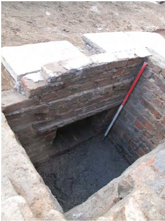
Figure 58: Ventilation access to (166).
