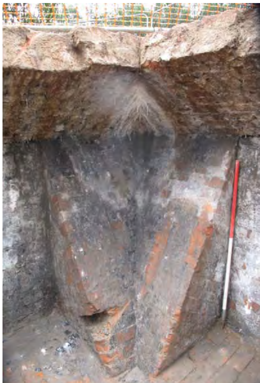
Figure 7: Detail of buttresses (143) at the (141) south-east corner of the retaining wall, looking south-east.
