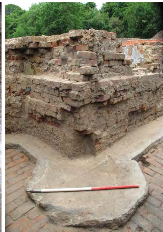
Figure 8: Detail of plinth projection at the eastern end of Corridor wall 5, looking east.
