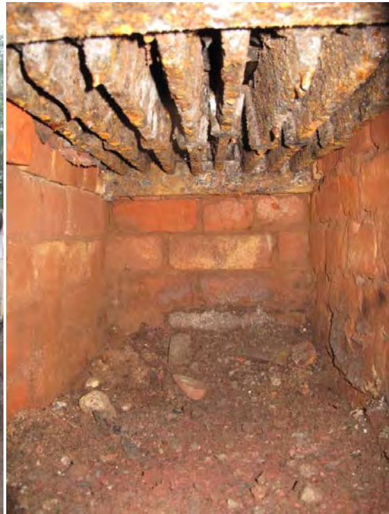
Figure 63: internal view of boiler (240 ) Within Room B14.
