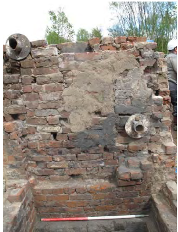
Figure 59: External wall and pipework of the heat exchange.
