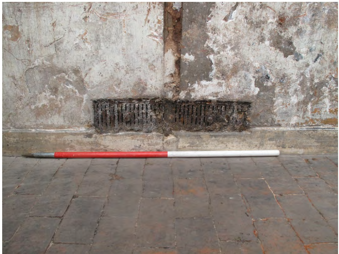
Figure 54: Cast iron ventilation plates leading to the heat exchanger (253) within Room B12.
