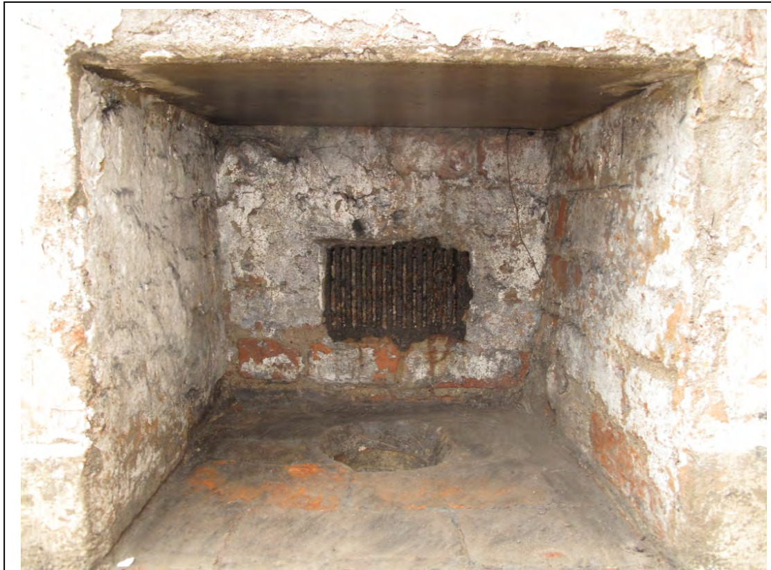
Figure 53: Access point to heat exchanger (253) within Room B12.
