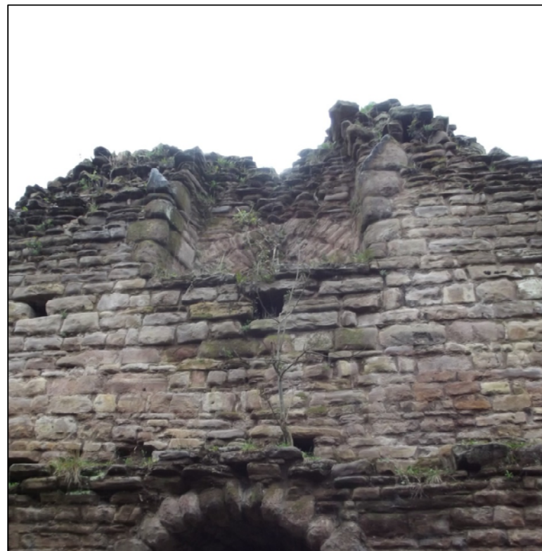
Fig 39: The interior corner of Radcliffe Tower, looking at the fireplace above the archway in the western elevation. Note the arch to the top of the fireplace and the chamfered surrounds. Note the four redundant beam slots from the 19 th century use as a barn.
