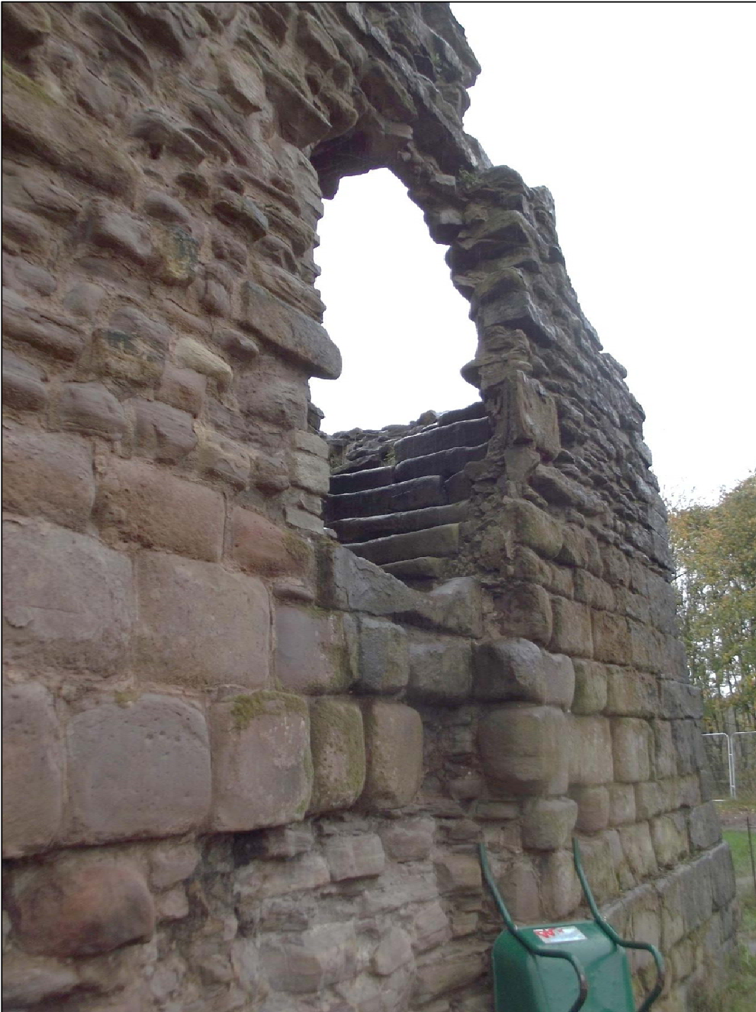
Fig 44: The first floor doorway to the tower in the western elevation. Note the surviving stairs.
