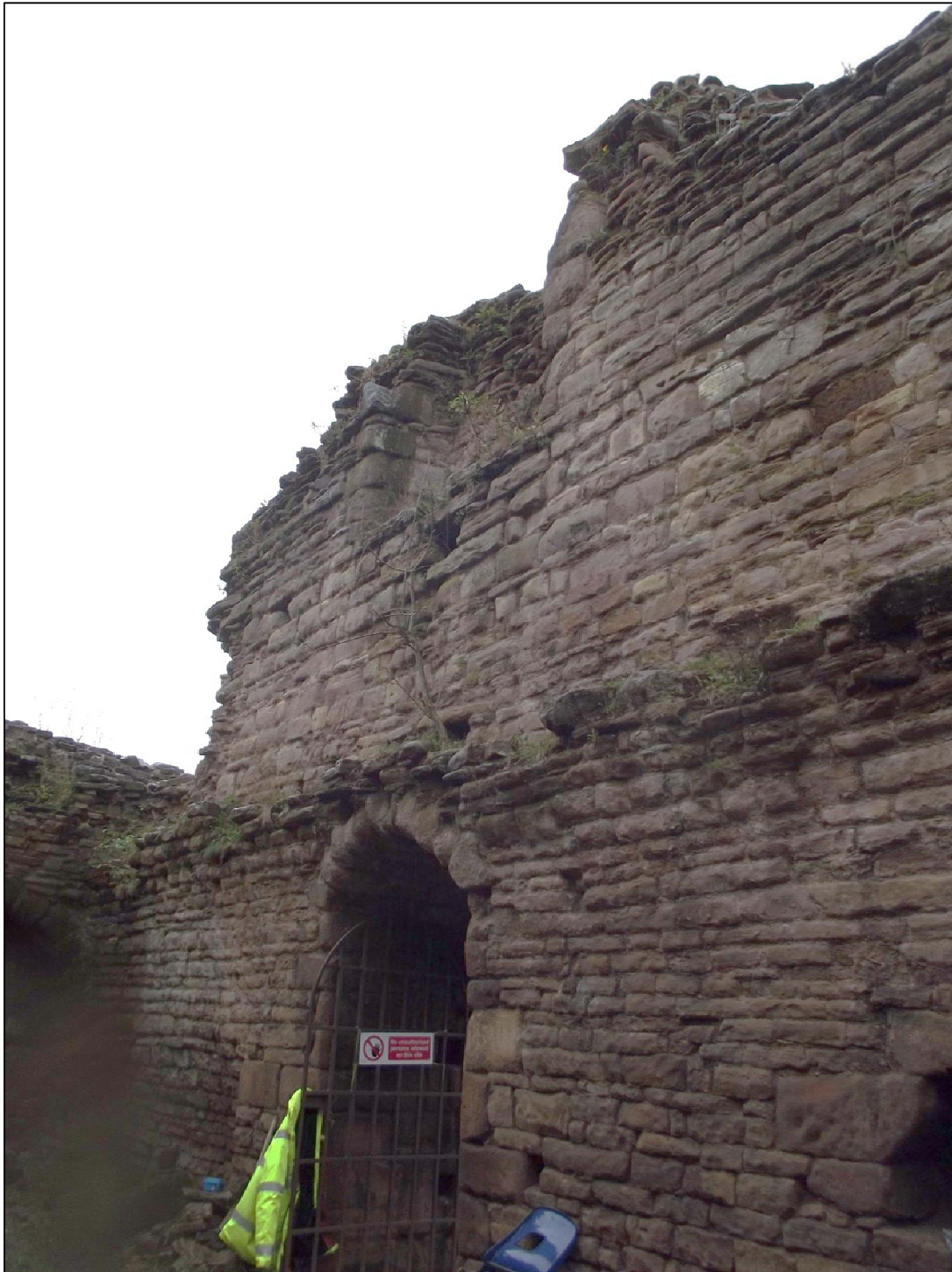
Fig 43: Interior of Radcliffe Tower, looking at the inner western elevation with the remains fo the barrel vaulting and the first floor fireplace.
