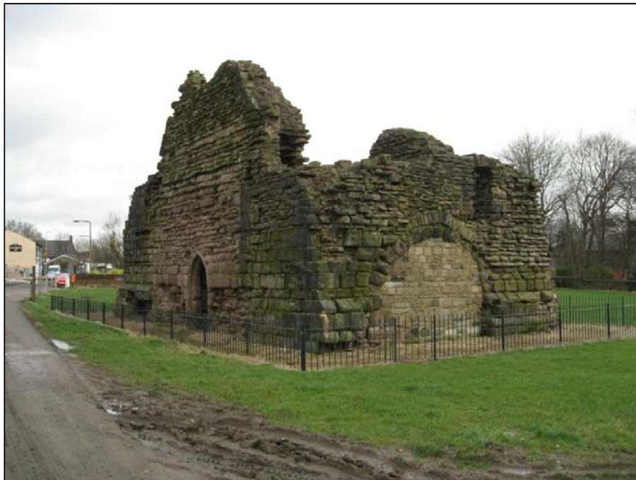
Fig 25: The western and southern elevations of Radcliffe Tower in 2008. The haulage road is to the left.
