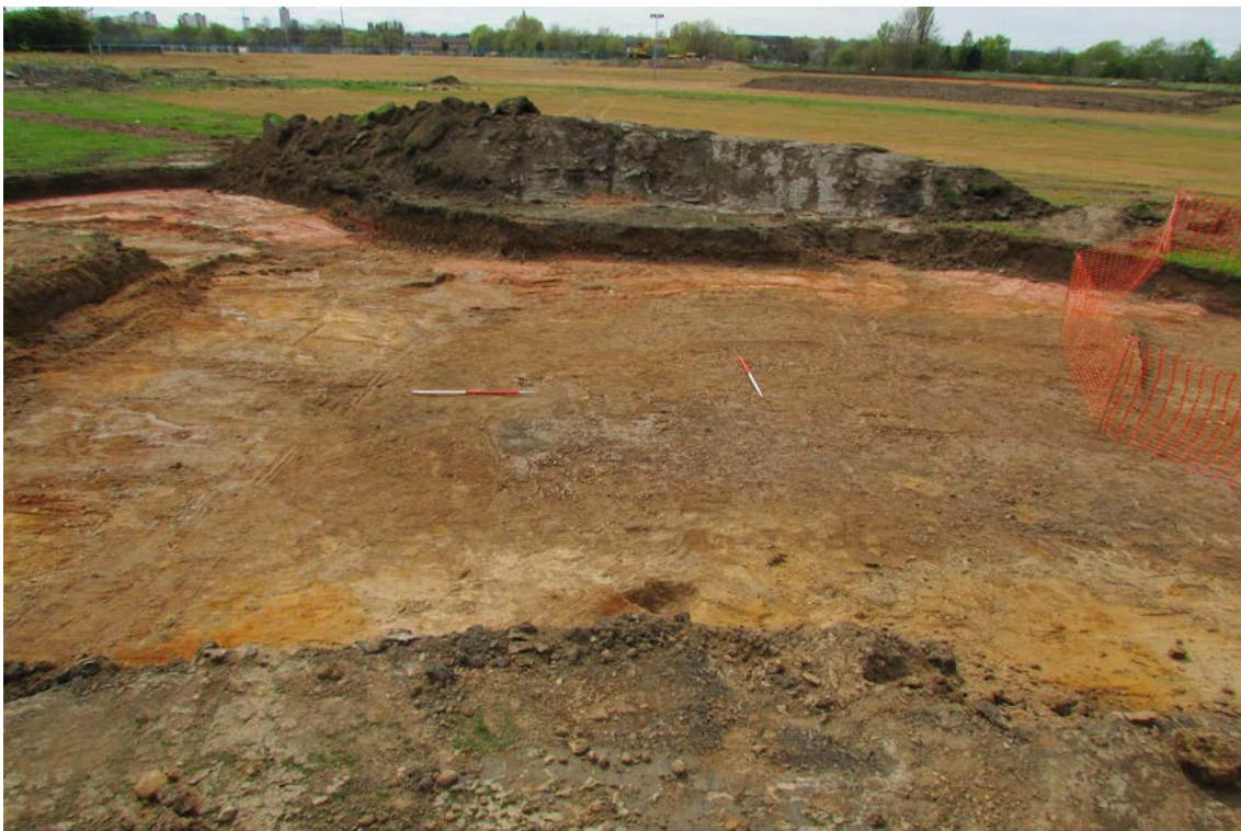
Fig 21. Fill (124) showing the terminus (pre-excavation) against the natural red sandstone (108) in the background and the sands and gravels (107) in the foreground.
