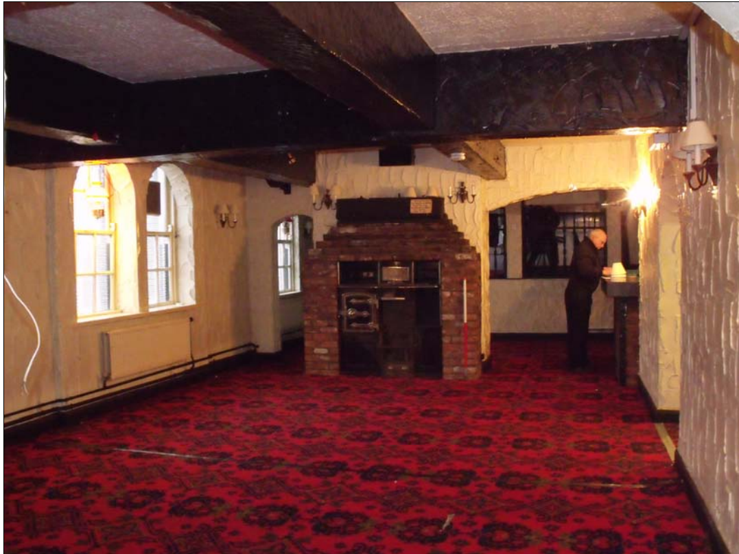
Fig 12: George & Dragon Hotel room FF6 looking eastward towards room FF7 and the site of the new staircase behind the inserted fireplace.
