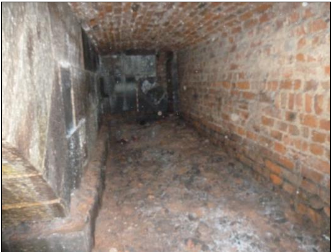
Fig 23: View of Room C19 looking south with a stone arch to the left.
