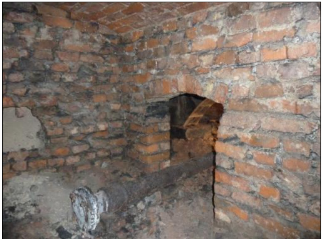
Fig 7: View of the Room C1 looking south-east showing a heating pipe.
