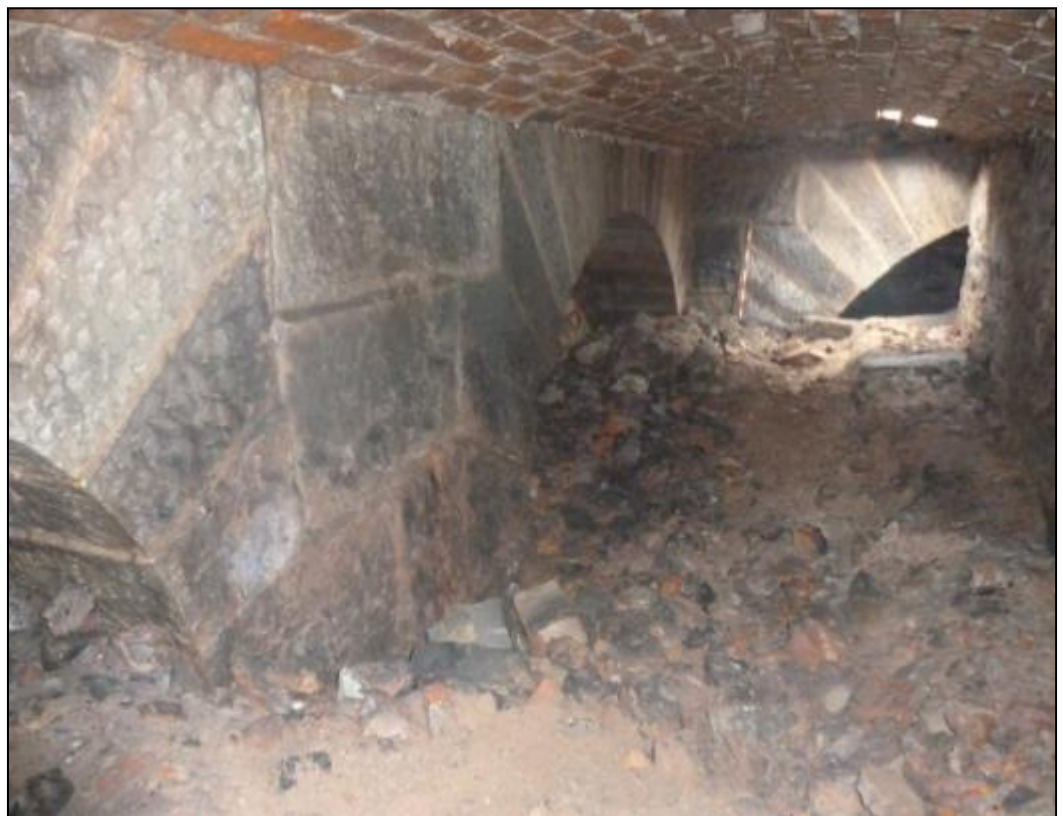
Fig 29: View of Room C27 looking north-west with stone arches in the background and to the left, and rubble-strewn floor.
