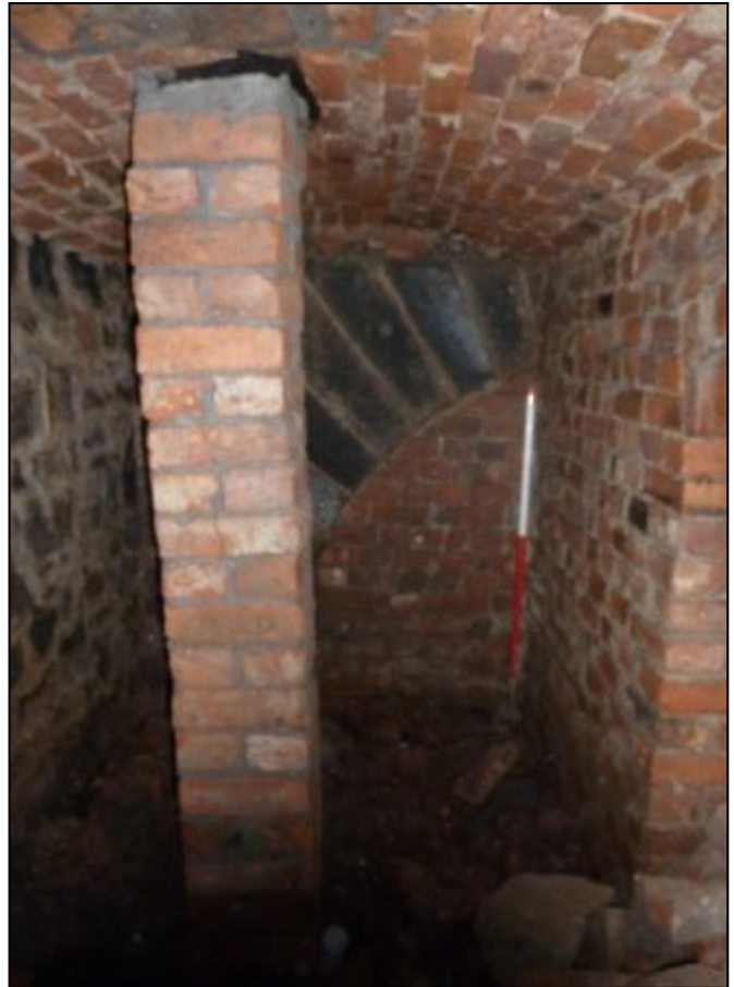
Fig 28: View of Room C26 looking north at an inserted machine-made brick pillar supporting the barrel vaulting. Note the stone arch behind.
