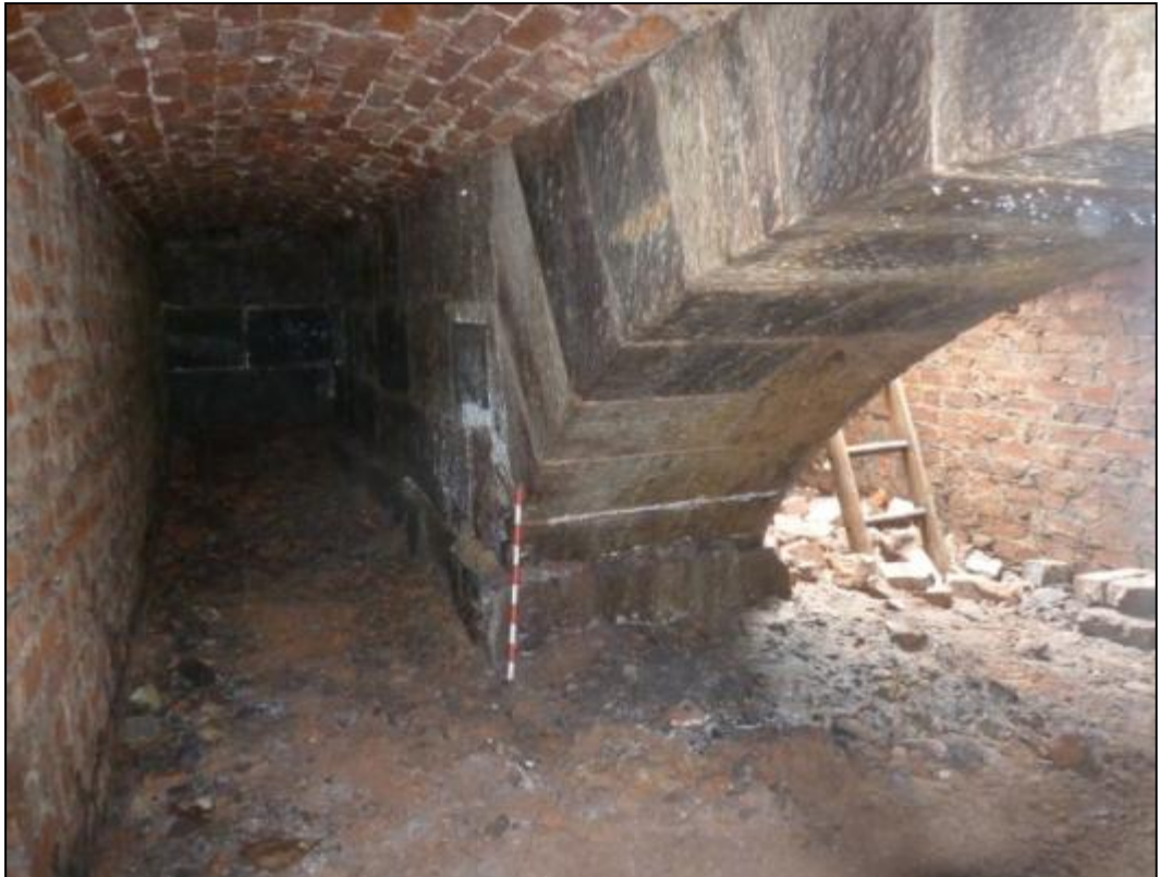
Fig 22: View of Room C16 looking south-west through a stone arch towards one the access points.
