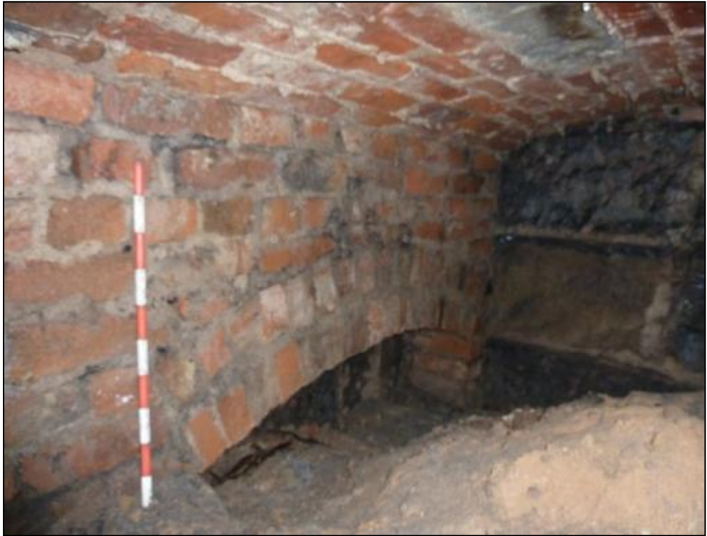
Fig 18: View of Room C11 looking south at a brick archway and what appears to be an inserted iron beam on the right.
