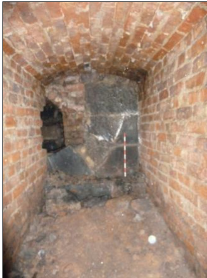
Fig 21: View of Room C13 looking at the southern wall and another inverted stone arch.
