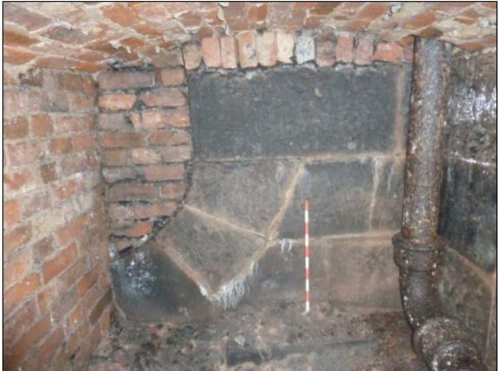
Fig 10: View of Room C4 looking at the southern wall showing a blocked stone inverted arch and heating pipe to the right.
