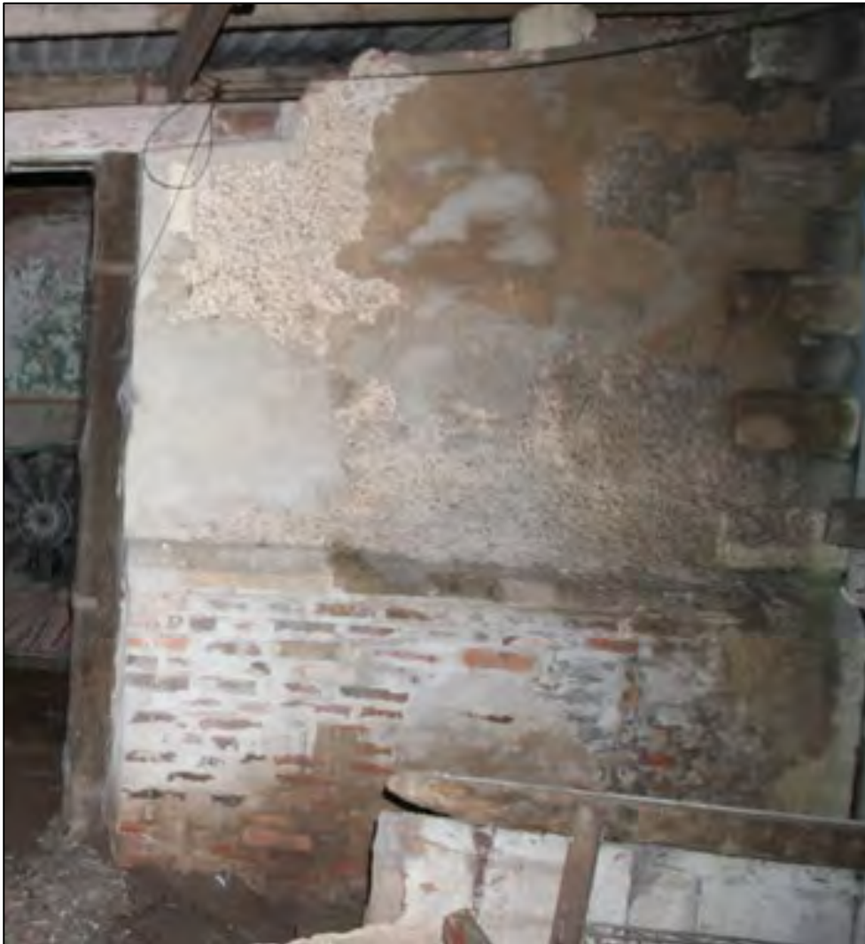
Plate 26: Southern part of the east wall of Room G8, with refaced brickwork and rusticated quoins
