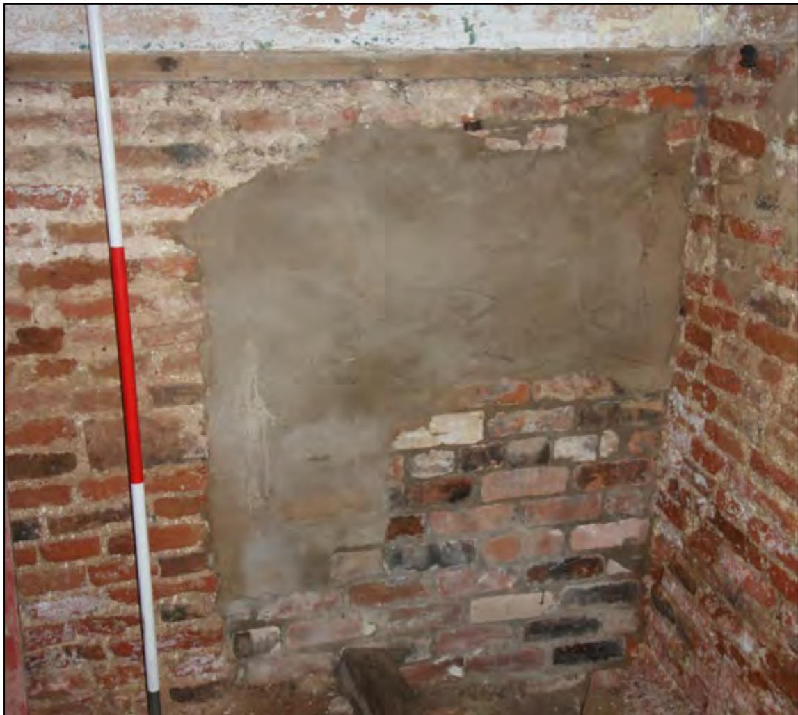
Plate 37: Detail of blocked doorway at east end of north wall, Room G1
