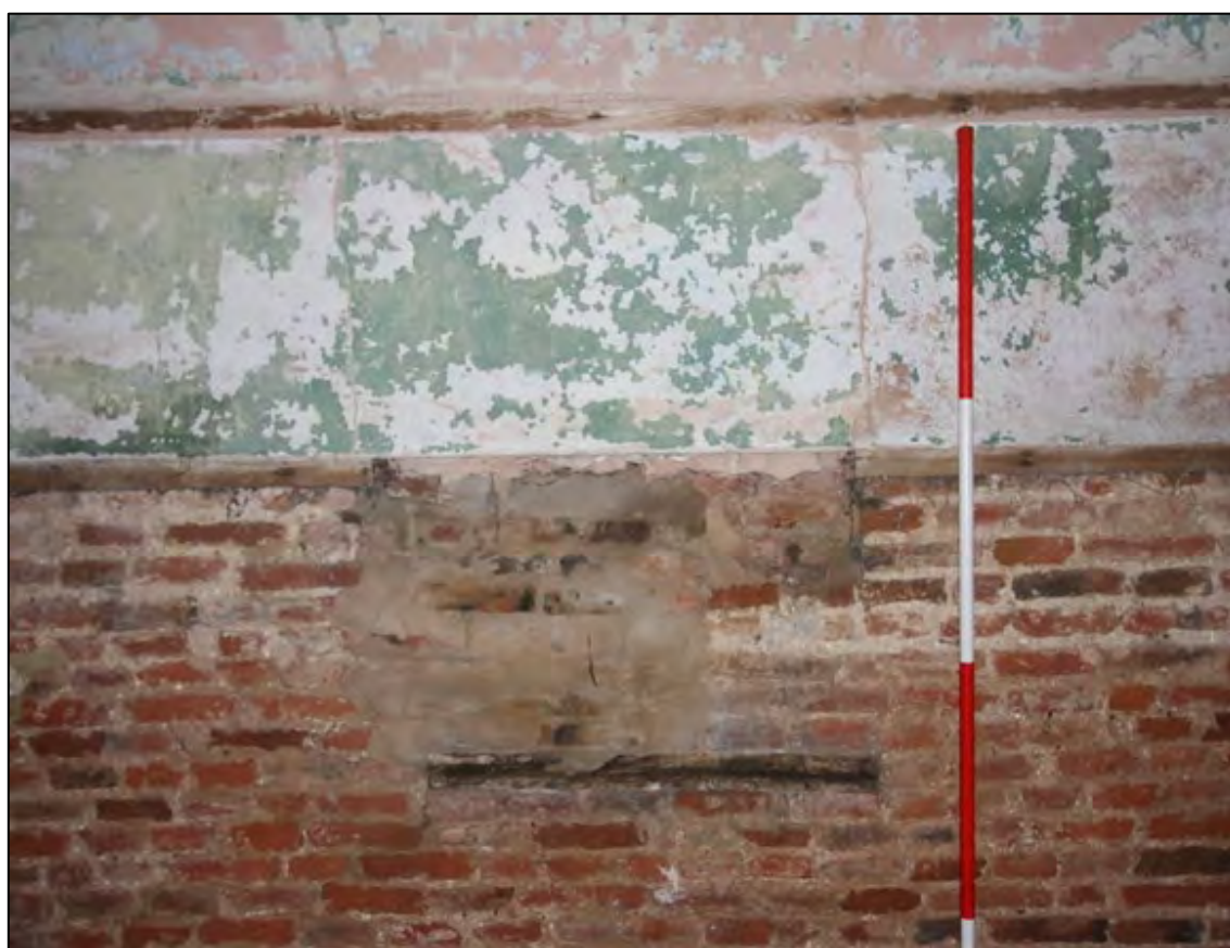
Plate 38: Blocked window spanning floor levels within the post monastic house, Room G1
