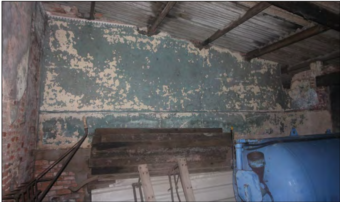
Plate 46: South wall of Room G2, with large timber pile obscuring central area
