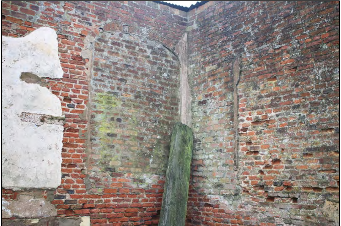
Plate 21: Blocked doorway and picture window at the return of the central section of the north wall
