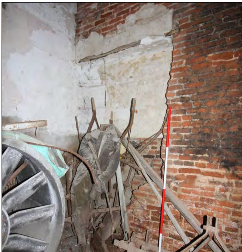
Plate 34: Alcove at the east end of the south wall, Room G1, with blocked doorway obscured by farm machinery
