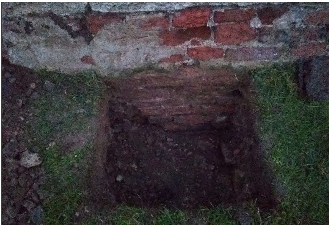
Plate 66: Detail of trench 3, showing deterioration of wall face
