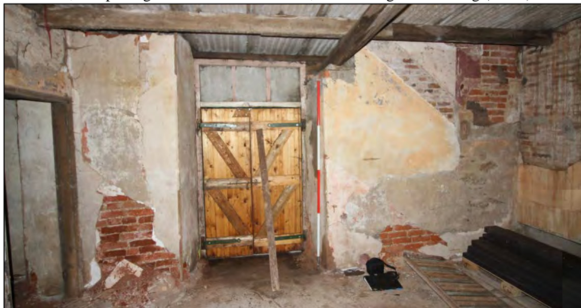
Plate 49: South elevation of Room G3, with scar for stairs and maroon-coloured plaster
