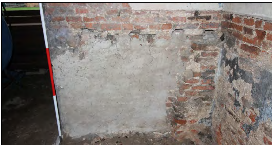
Plate 40: Lower part of west wall, with projecting stub and infilled window, Room G2
