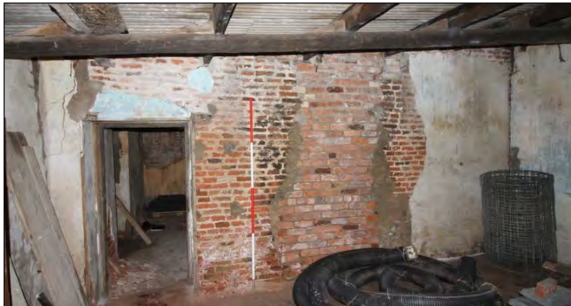
Plate 58: West elevation of Room G4, with inserted doorway and removed and blocked chimney breast
