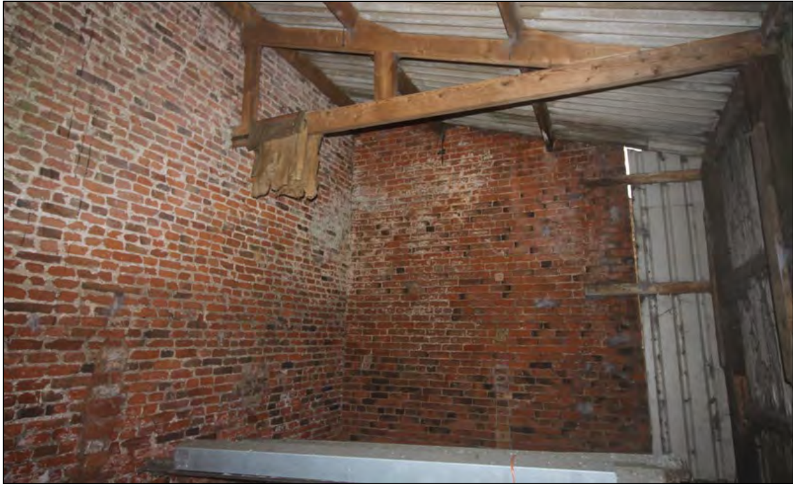
Plate 60: Detail of roof truss and vertical wall scars for internal walls, G6
