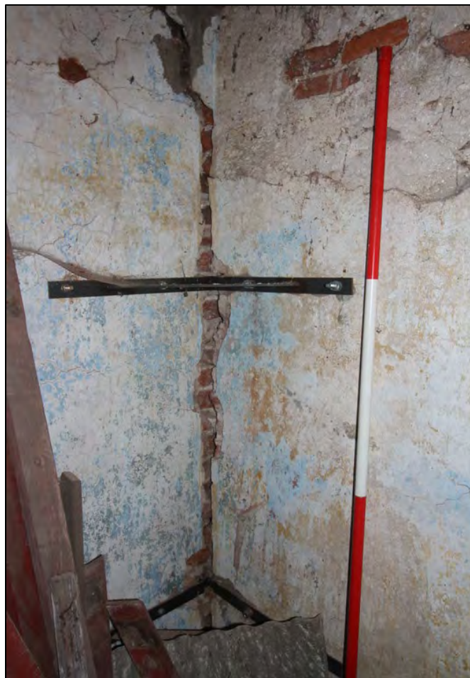
Plate 56: Modern wall ties across junction of east and south walls, Room G4
