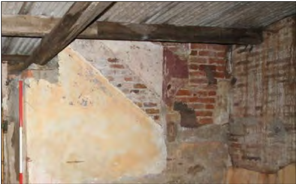
Plate 51: Misaligned brickwork at junction of south and west walls, with scar for stairs, Room G3
