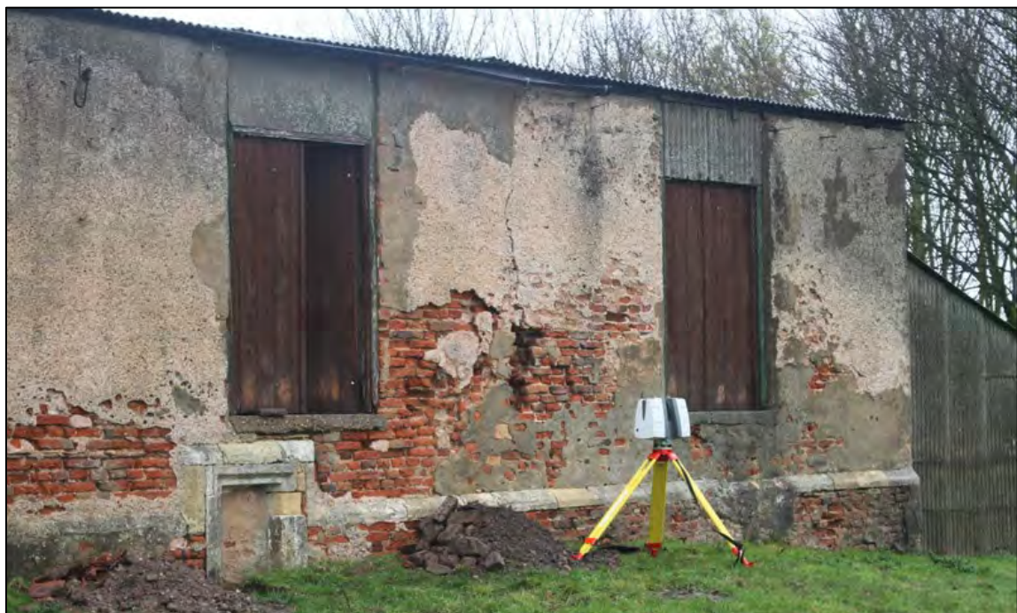
Plate 14: Eastern element of the southern façade, with blocked window partially below present ground level
