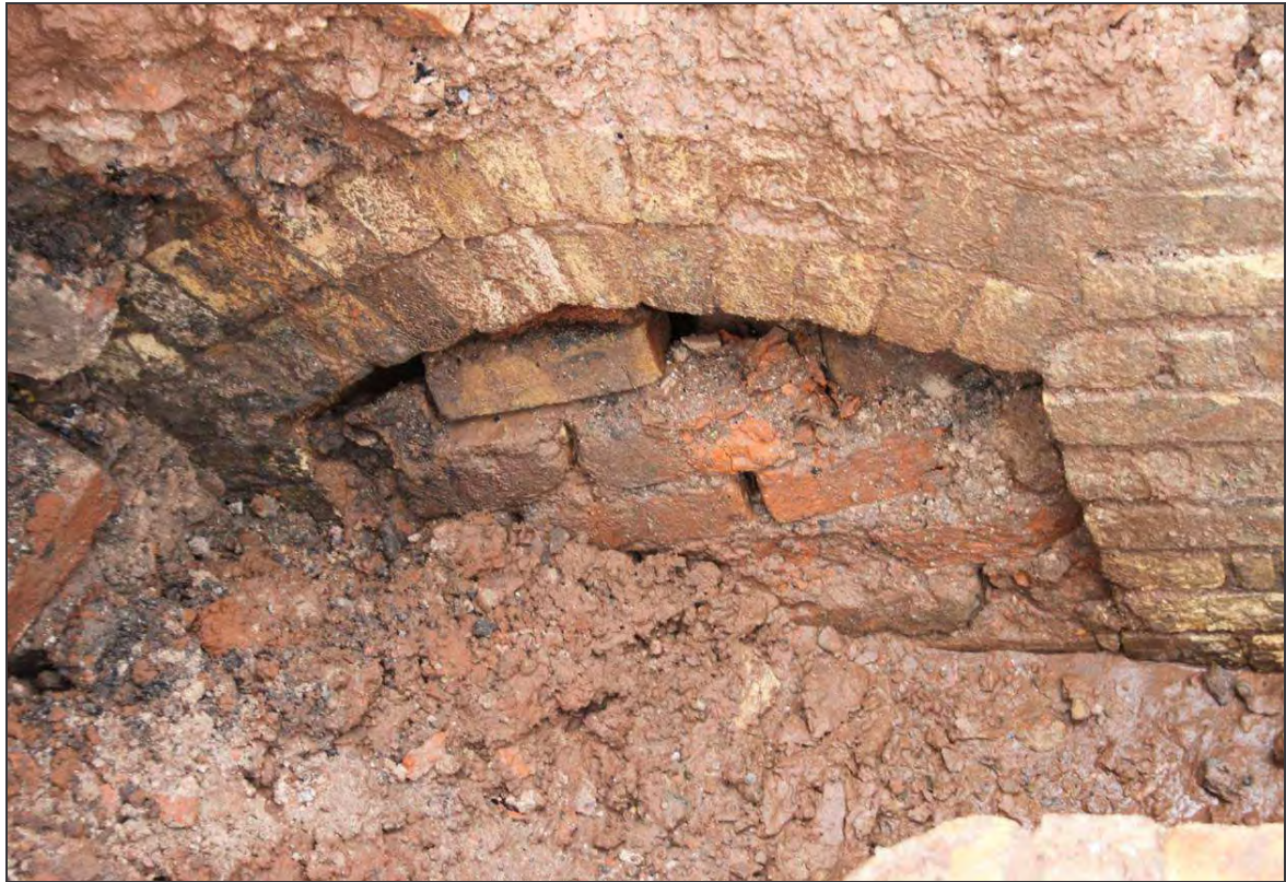
Plate 6: Blocked aperture within the north wall of the flue leading to the north boiler house
