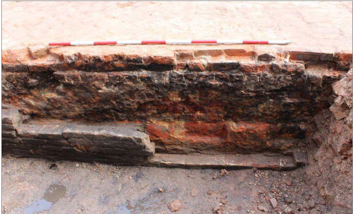
Plate 17: West elevation of the chimney showing exposed courses of stone base, partially obscured by a later skin of firebrick (2m scale)
