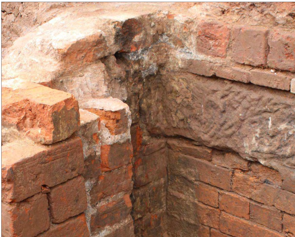
Plate 12: Detail of rebated stone block. Note the tile packing added below the stone.
