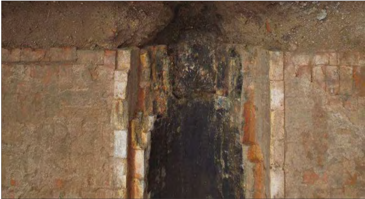
Plate 23: Ramp at southern end of horizontal flue, beginning within the chimney base
