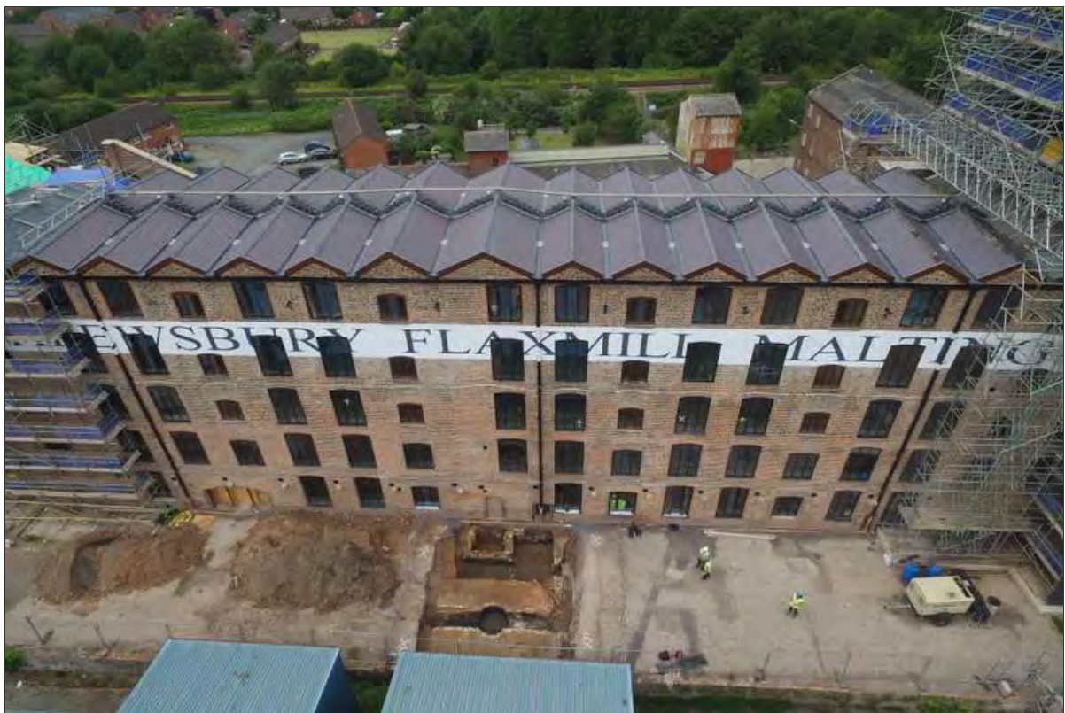
Plate 32: General view of the east face of the Main Mill, with the excavated privy tower and chimney base in foreground
