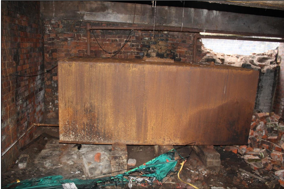
Plate 14: The mild steel diesel tank at the north-eastern end of the boiler house
