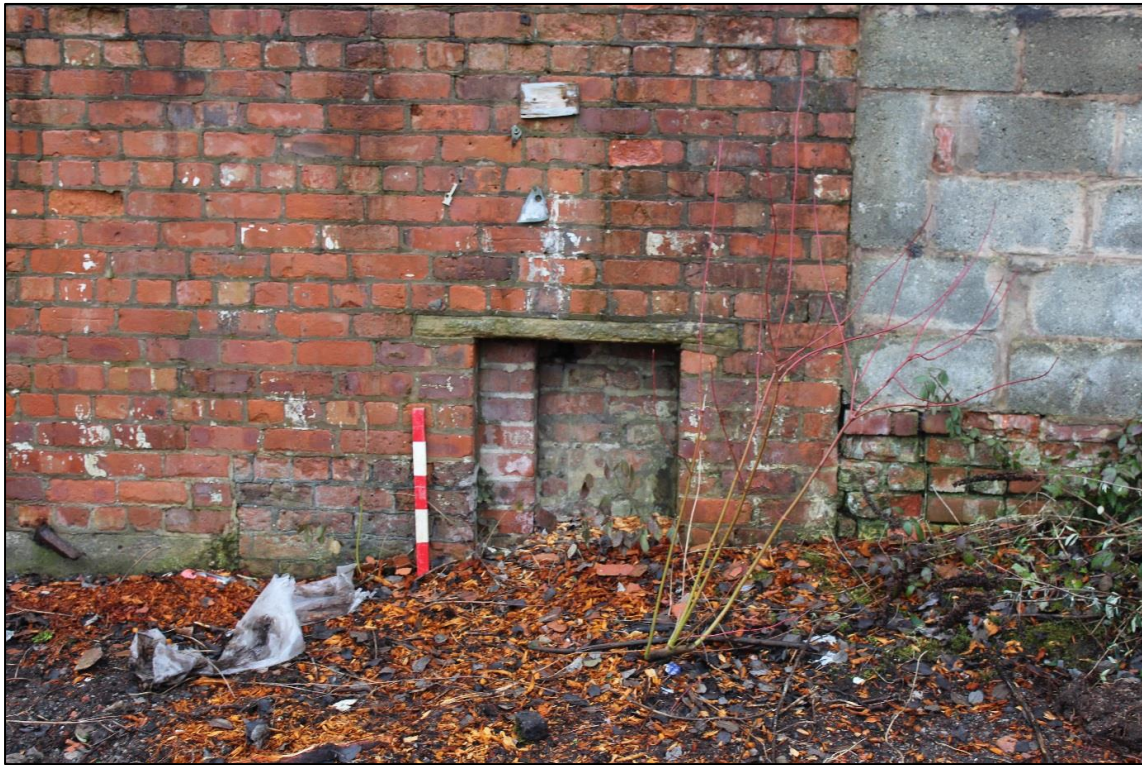
Plate 7: Detail of cut out in the wall for pipework leading to the engine house
