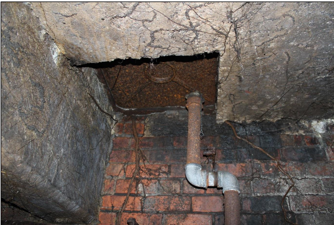
Plate 15: The manhole cover and 2" pipe from the diesel tank leading to the first floor of the boiler house
