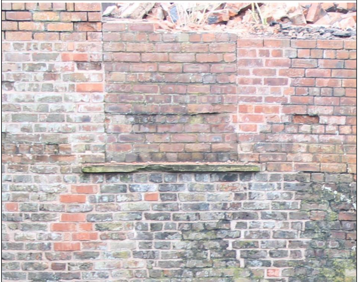
Plate 10: Detail of the blocked up window on the extended upper floor of the north-eastern façade, with earlier fabric on the left side of the jamb
