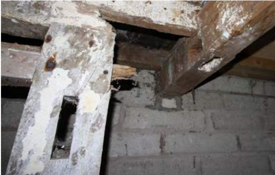
Gleaves Hill Barn 157: Mortice in hay feeder and further mortices in ceiling beam for stalling. Note the chamfer to the ceiling beam that stops before the post position
