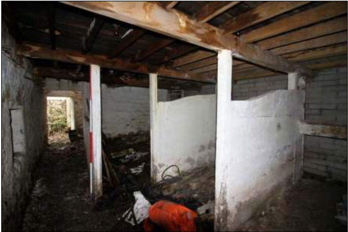
Gleaves Hill Barn 144: Replaced clinker block stalling in northern cowhouse, retaining timber posts
