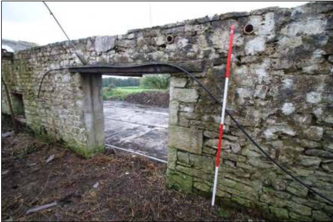
Gleaves Hill Barn 111: Quoined doorway in west wall of single-storey cowhouse extension
