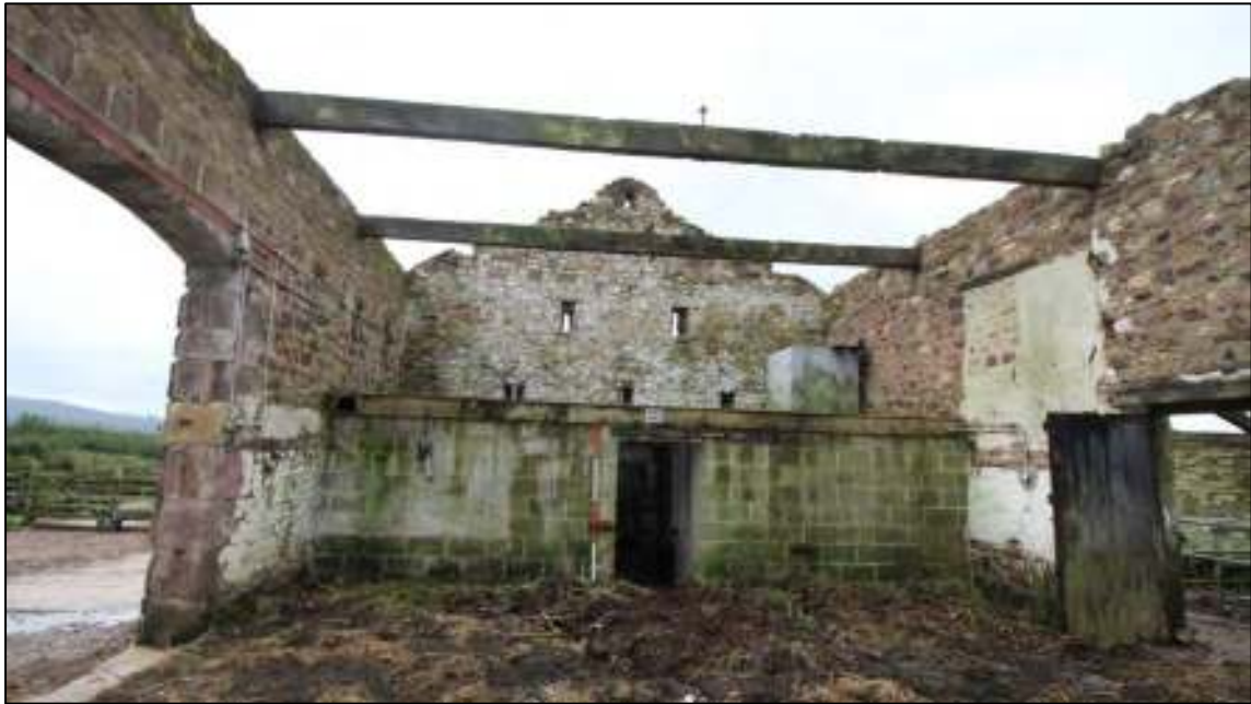
Gleaves Hill Barn 77: Ruinous threshing barn, looking south-west
