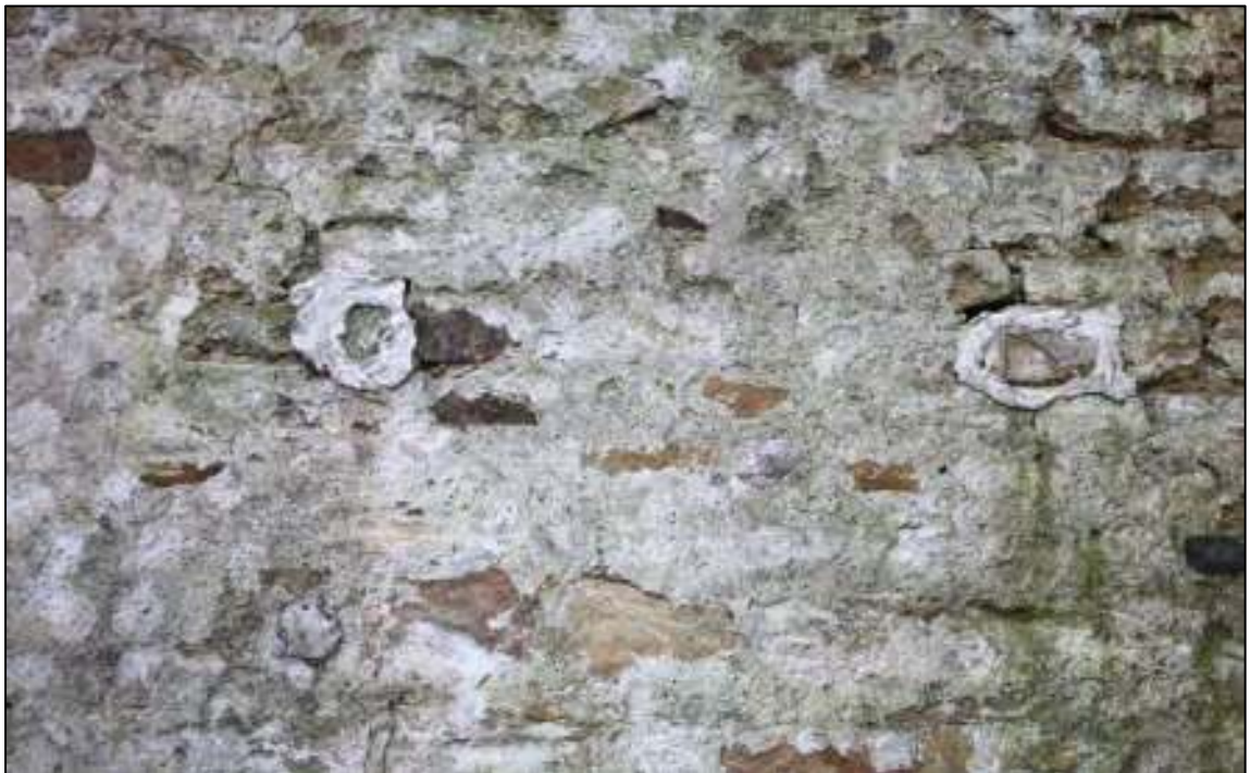
Gleaves Hill Barn 126: Blocked floor joist sockets for loft of single-storey outshut
