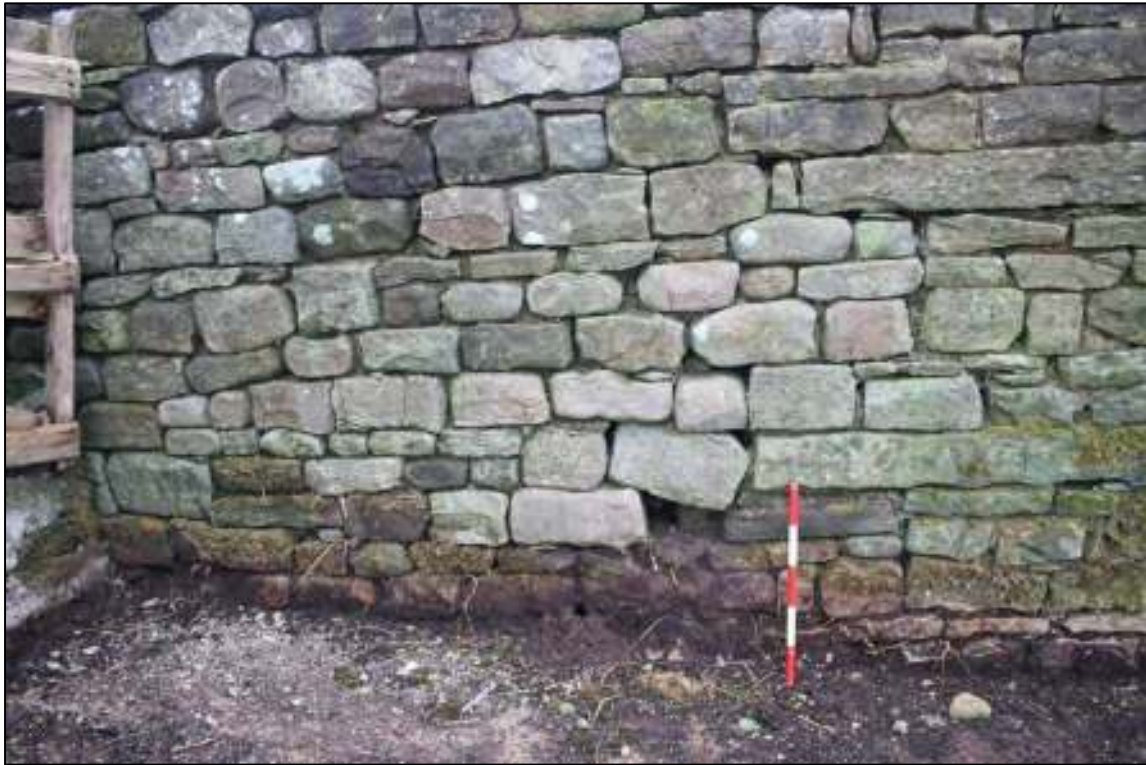
Gleaves Hill Barn 45: Drain aperture in base of west wall of single-storey outshut
