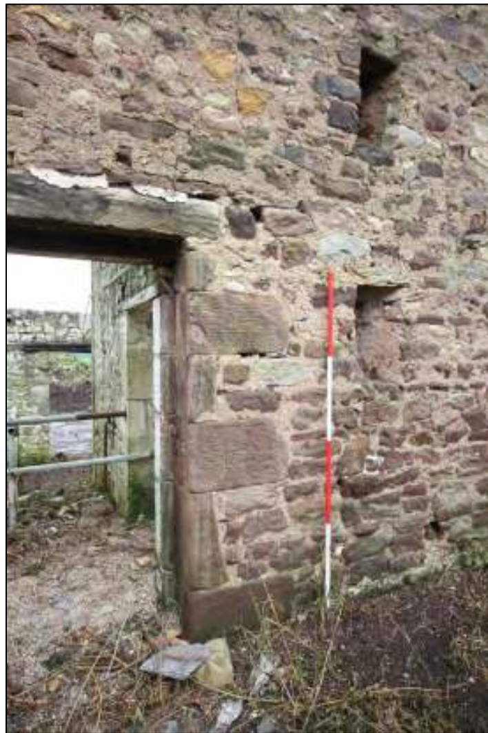
Gleaves Hill Barn 84: Quoined door jamb of winnowing door in west wall
