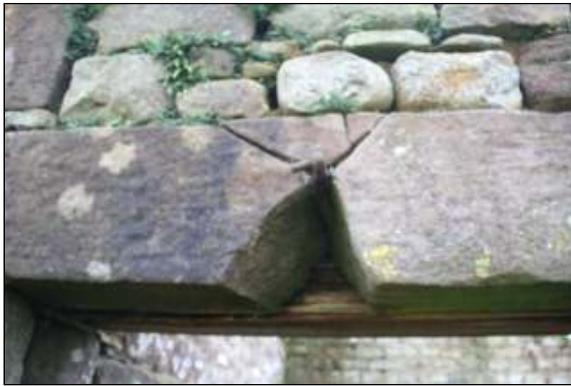
Gleaves Hill Barn 31: Detail of cracked door lintel
