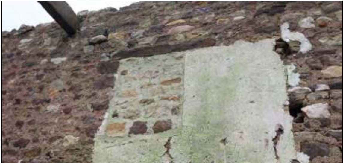
Gleaves Hill Barn 97: Blocked aperture above winnowing door in west wall
