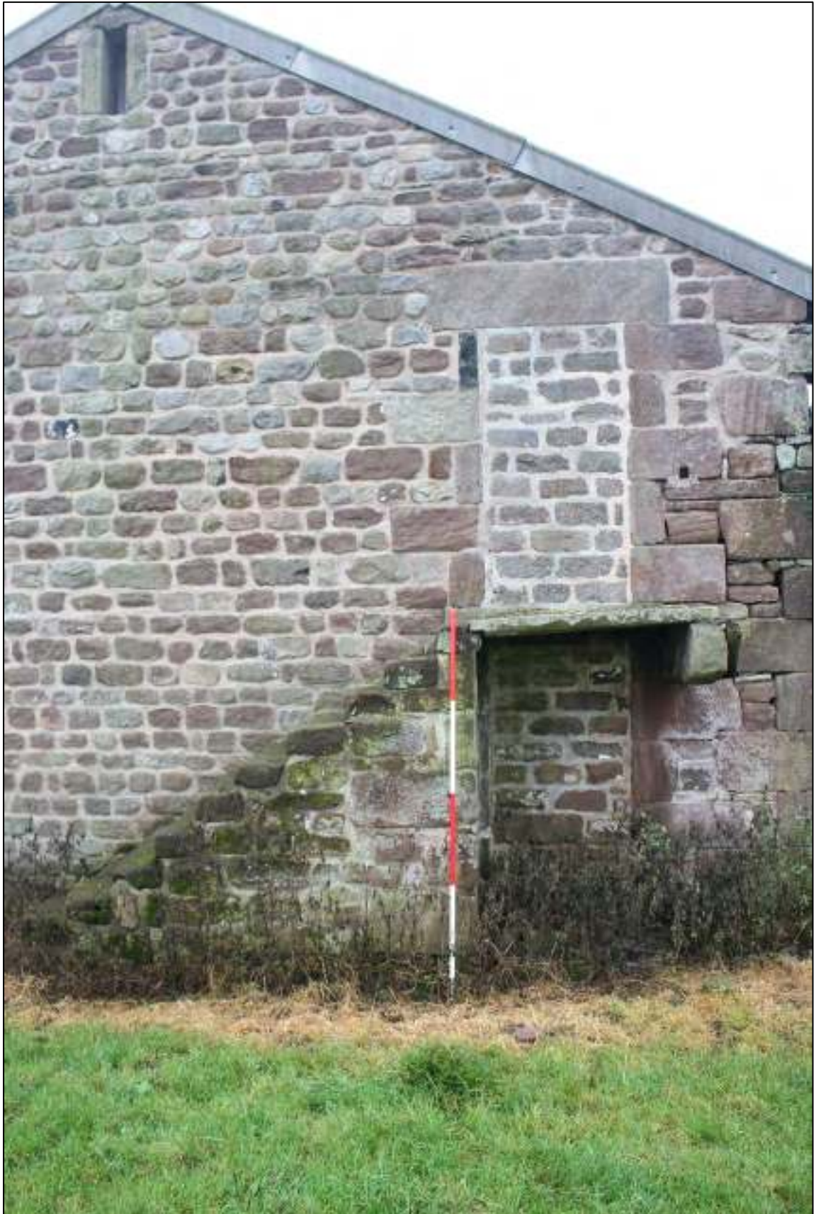
Gleaves Hill Barn 20: Blocked doorways and stairs, north gable
