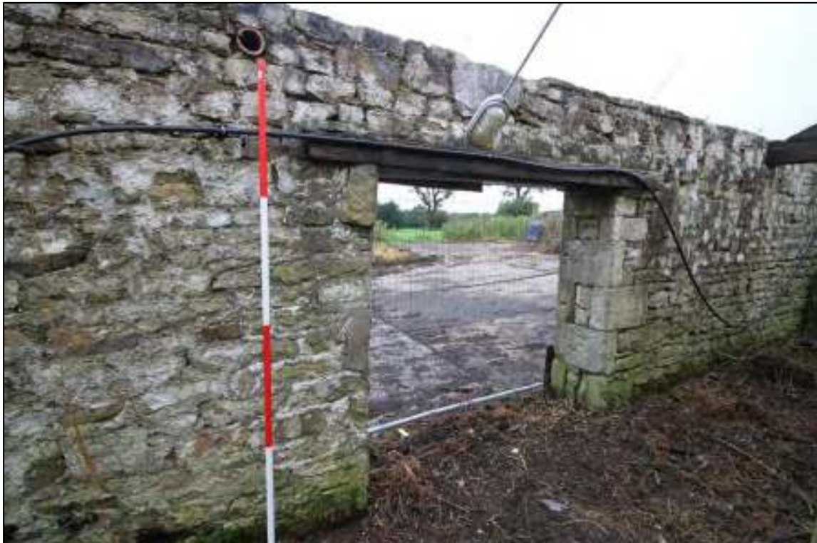
Gleaves Hill Barn 120: Quoined doorway in west wall of single-storey cowhouse extension
