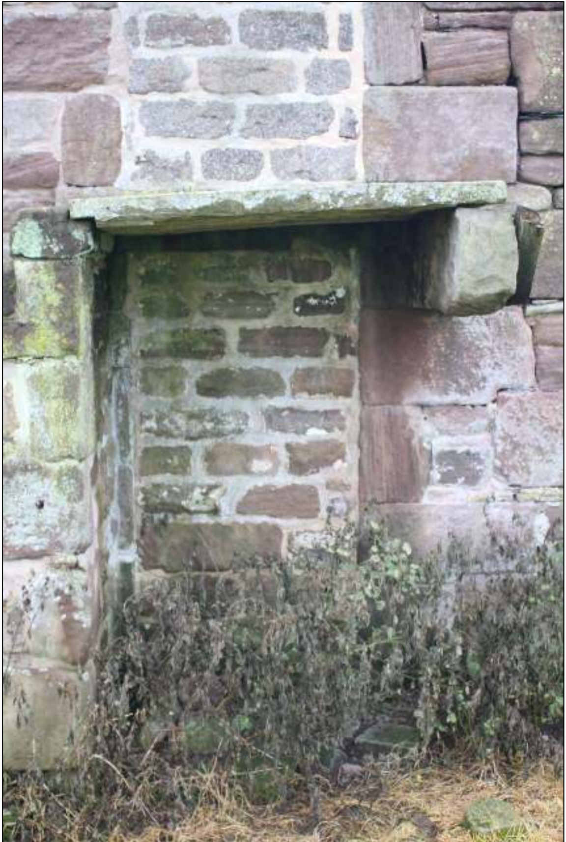
Gleaves Hill Barn 22: Detail of blocked lower doorway, north gable
