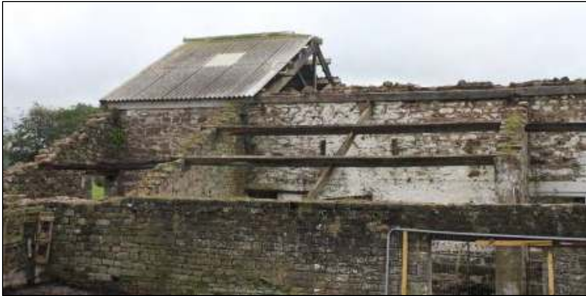
Gleaves Hill Barn 40: Roof structure of west extension, with original barn wall behind
