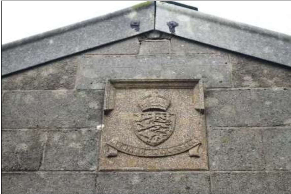
Gleaves Hill Barn 33: Cast-concrete Duchy of Lancaster coat of arms in gable of south extension, east face
