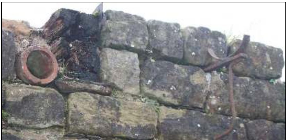
Gleaves Hill Barn 44: Detail of ceramic ventilator and cast iron-gutter bracket, west extension
