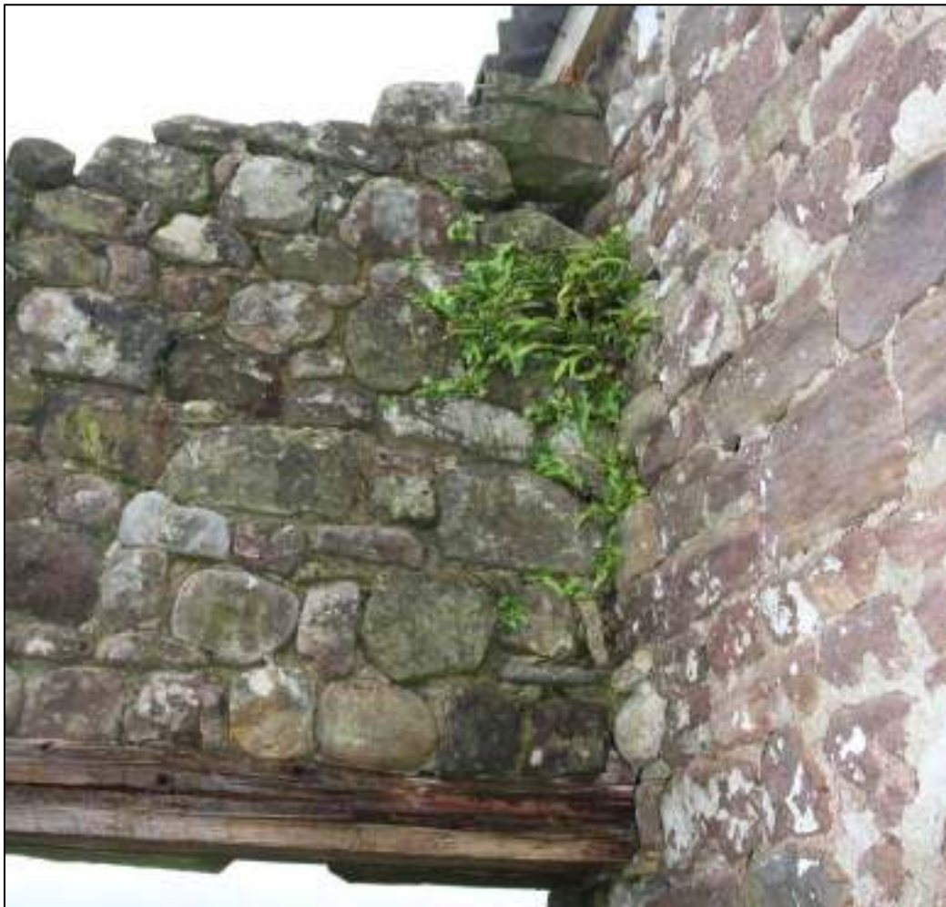
Gleaves Hill Barn 170: Lintel of door punched into earlier wall, with roughly-keyed wall above
