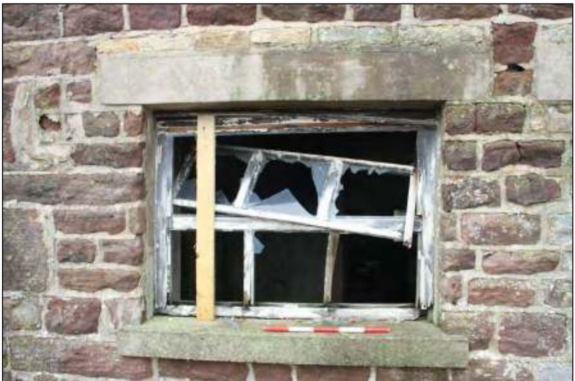
Gleaves Hill Barn 08: Detail of damaged window
