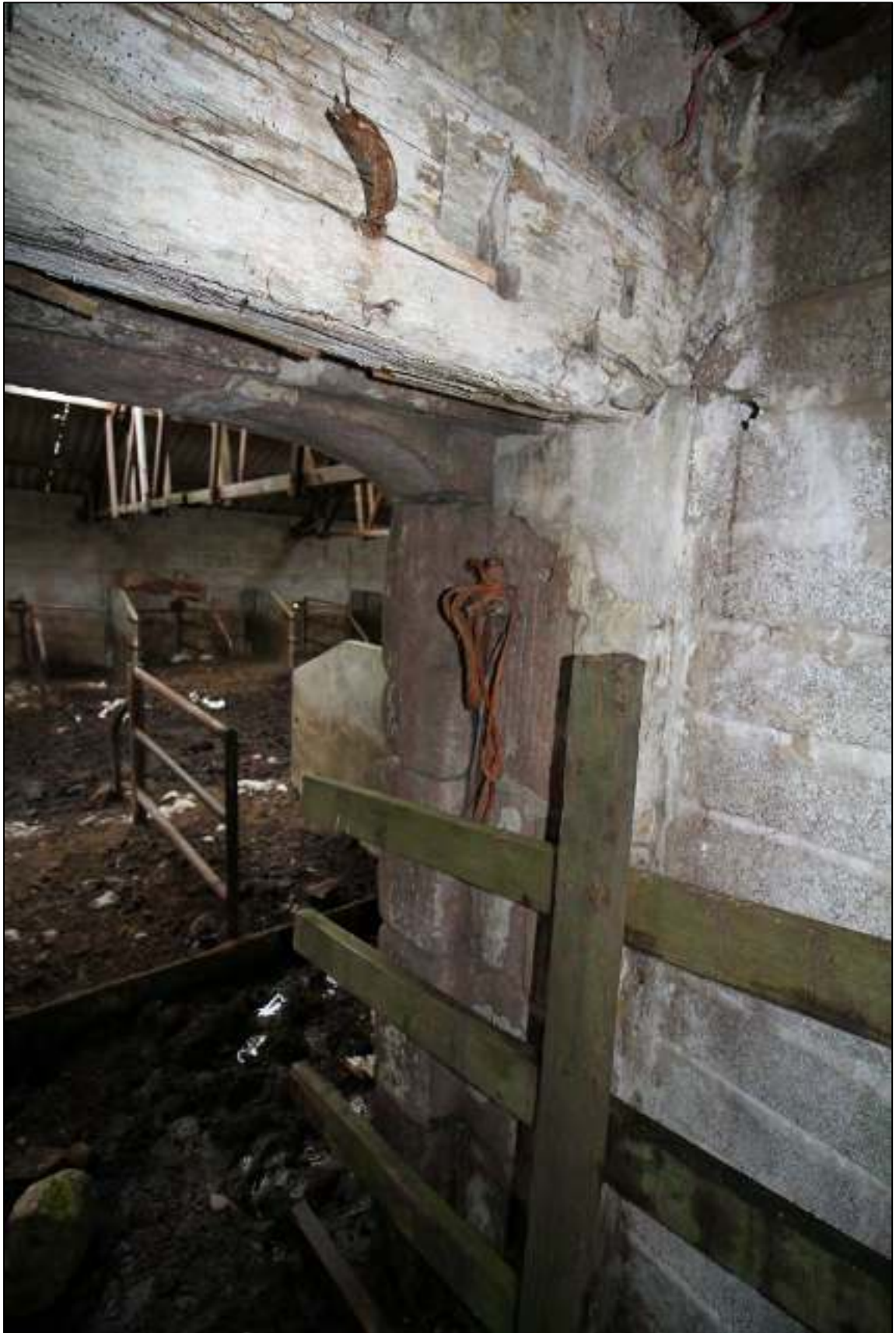
Gleaves Hill Barn 72: Detail of rebated stone jamb of central doorway in southern gable
