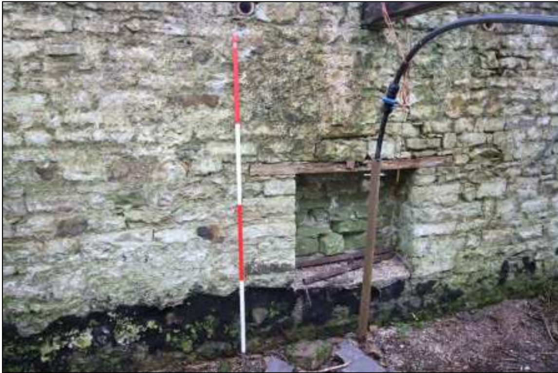
Gleaves Hill Barn 115: Keeping hole in west wall, of cowhouse extension
