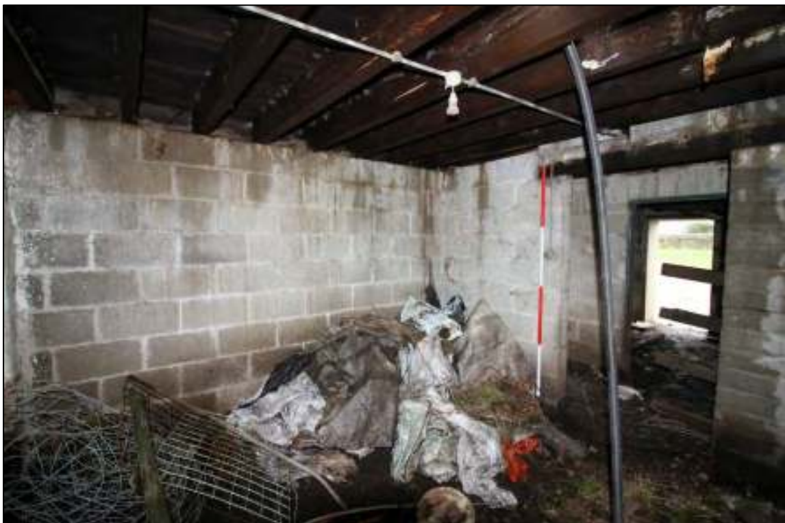
Gleaves Hill Barn 65: South cowhouse of original barn, looking east at rebuilt clinker-block walls
