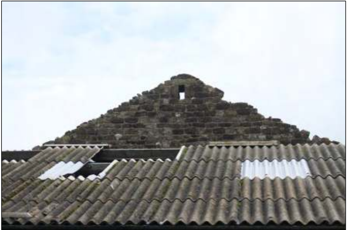
Gleaves Hill Barn 35: South gable of original barn, with owl hole, above late extension
