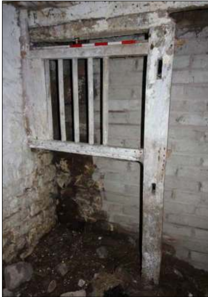
Gleaves Hill Barn 153: Detail of hay feeder, with mortices for rails of stalling
