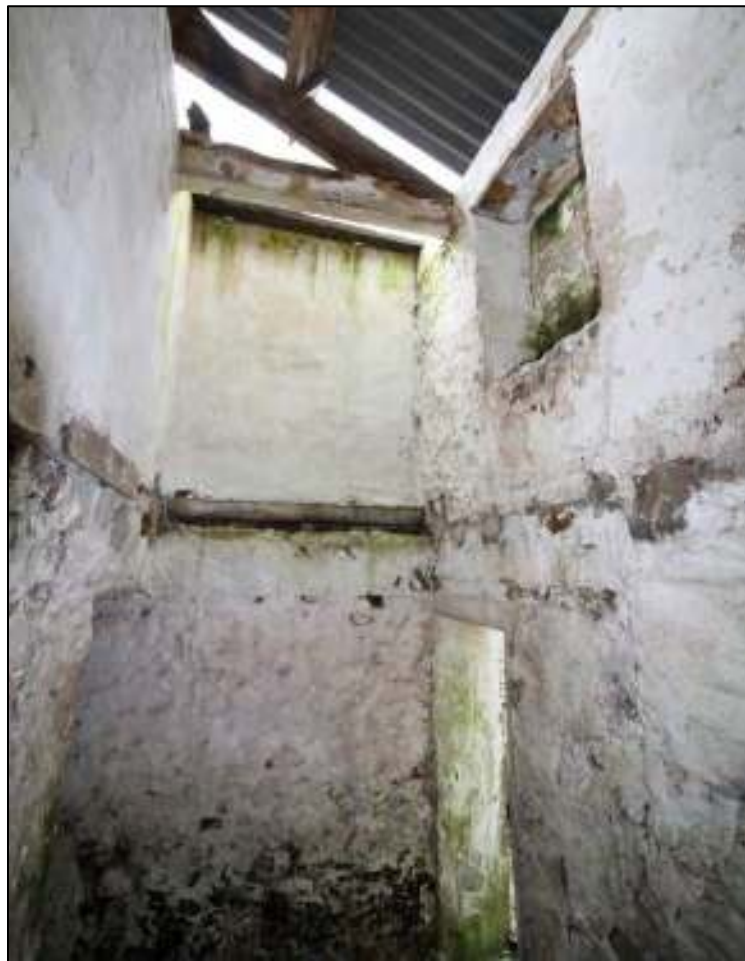
Gleaves Hill Barn 134: Small entrance passage in north-west corner of original barn, looking south-west
