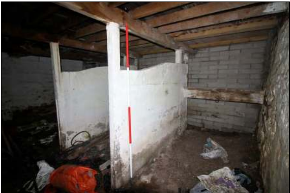
Gleaves Hill Barn 145: Detail of replaced clinker block stalling in northern cowhouse, retaining timber posts
