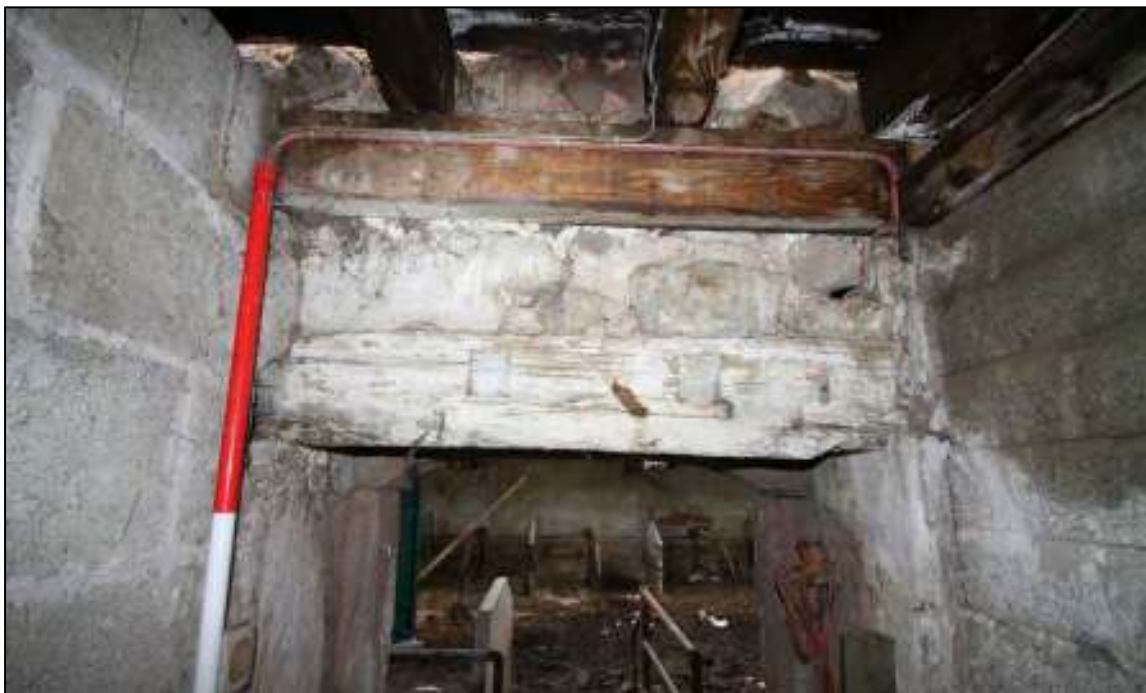
Gleaves Hill Barn 71: Internal lintel detail of central doorway in southern gable
