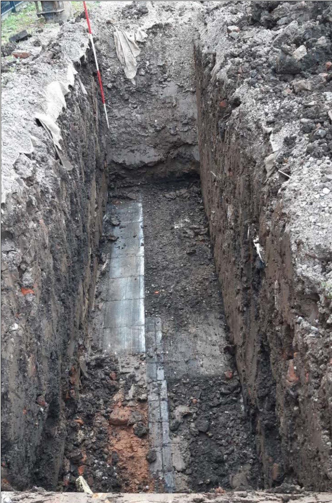
Plate 9: Trench 12, south-western end, showing engineering brick 013 in the centre with paving slabs 014 and sand 015 to the south-east
