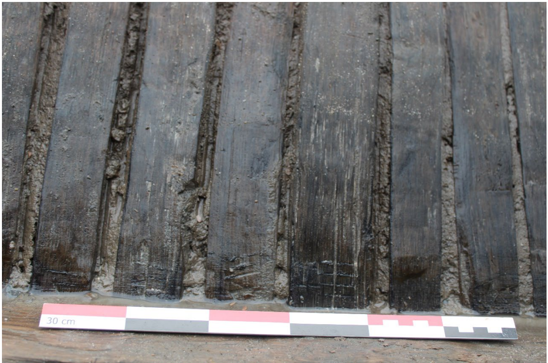
Plate 21: Trench B, an example of the assembly marks on the upright laths, bridge base frame [333], looking east, scale: 0.30m horizontal
