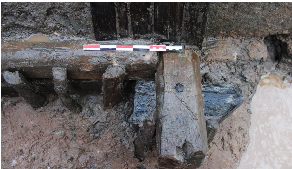
Plate 20: Detail of the lap-joint securing timbers [283]/[310] on the bridge base frame, scale: 0.30m horizontal
