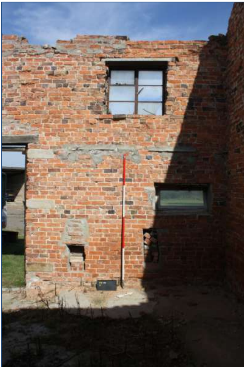
Plate 29: G1 possible alteration in north-west elevation to facilitate treashing machinery looking south-east.
