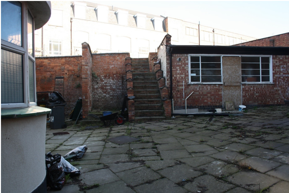
Plate 11: Outbuilding and steps to terracing to rear of Holly Bush Restaurant looking north east.
