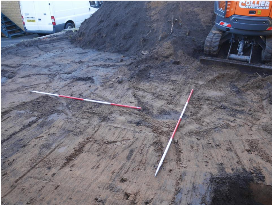
Photograph 2: View of the site after removal of the top soil, showing the natural sandy surface, facing southeast
