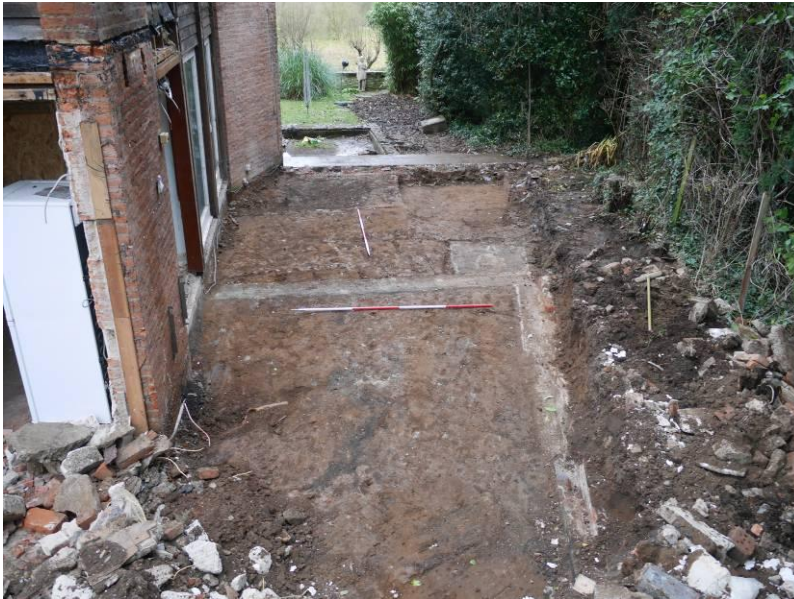
Photograph 2: View of the site after removal of the concrete ground surface, facing southwest
