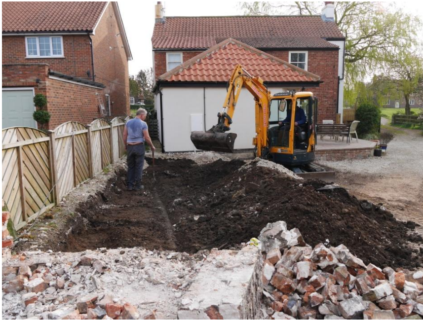
Figure 2: Image showing the excavation of the foundation for the new extension. Looking east
