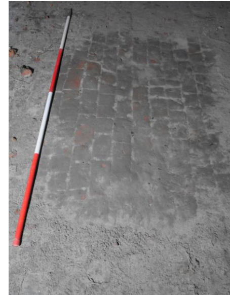
Figure 11: Heavily worn brick flooring inside the single nave barrel vaulted cellar
