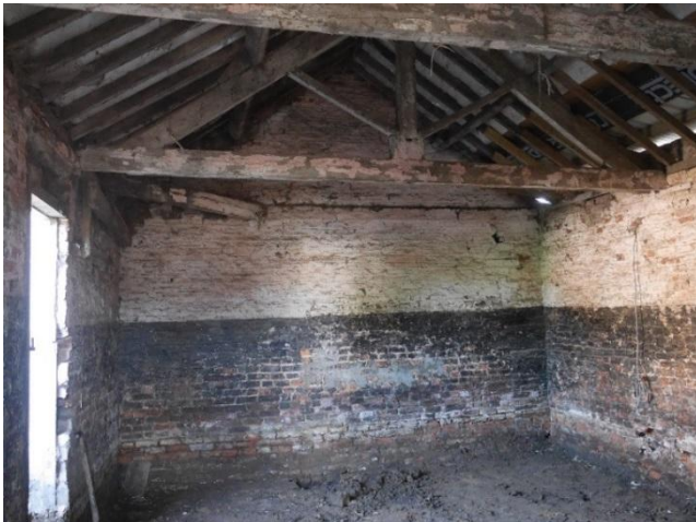
Figure 12: Details of the King Post Roof Construction Typical of All Three Buildings.
