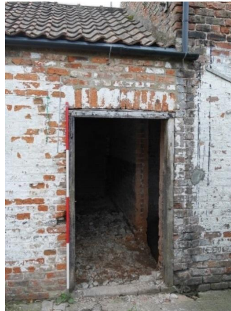
Figure 13: Loosebox West Facing Elevation Entrance. The door frame on the west facing elevation is constructed of timber with a single row brick lintel (Fig.17).
