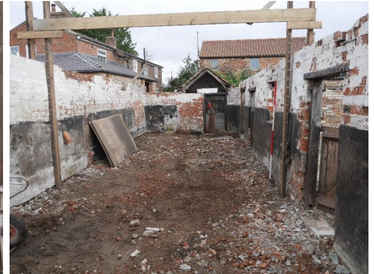
Figure 17: Internal aspect of the Cow House after the removal of the roof and concrete flooring.
