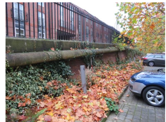
Figure 62: View of the retaining wall with decorative ashlar plinth and turned iron railings
