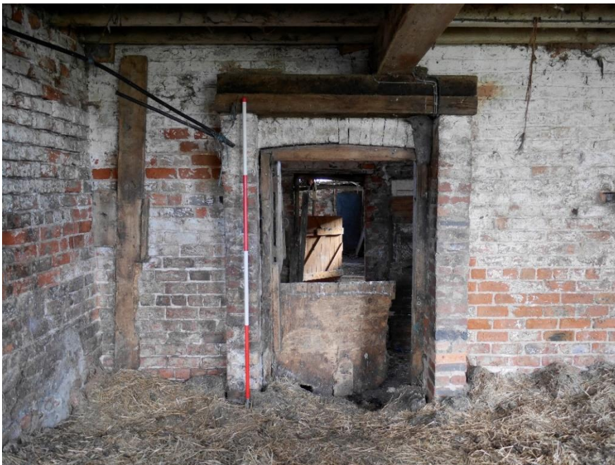
Image 11: Inside the Cart shed looking south through the single storey barn towards the doorway linking the Combination Barn to the Multi Bay Shelter Shed.
