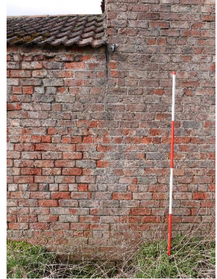
Image 13: East elevation of the Combination Barn and Shelter Shed with scarring due to an increase in height.
