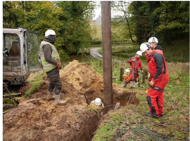
Figure 4: The replacement pole was installed at a depth of 2.80m below ground level.
