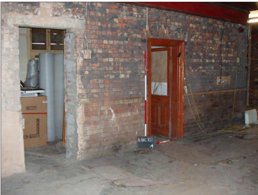
Photograph 15 Blocked Recess in Partition Wall (Scales 1 x 2m & 1 x 1m)
