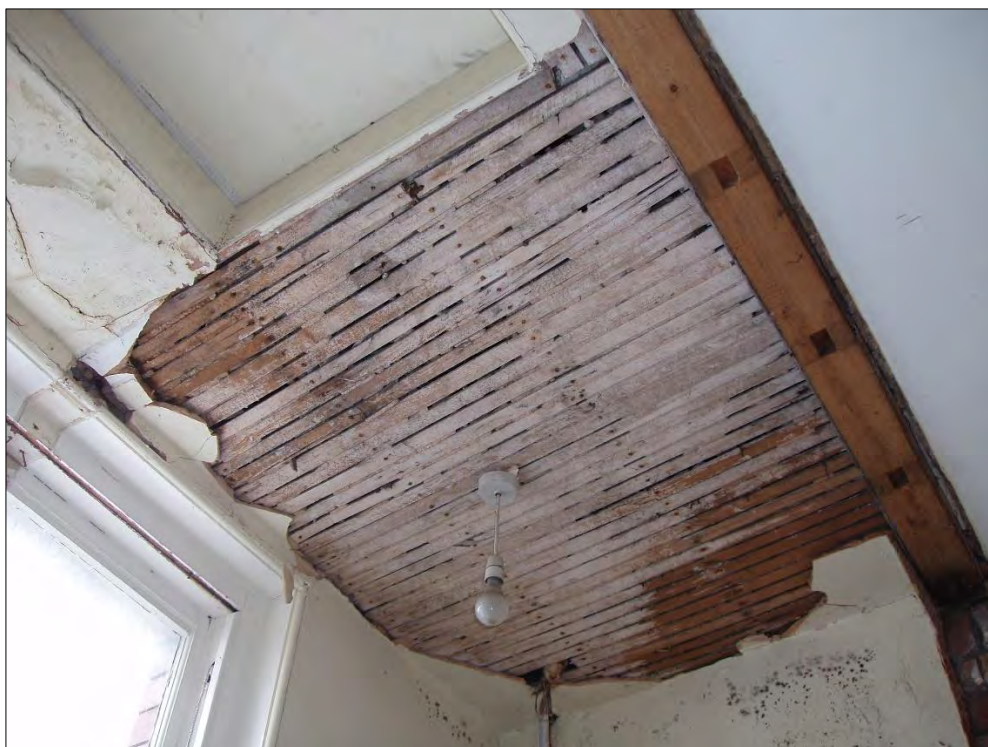
Photograph 32 Lathe and Plaster Ceiling Exposed
