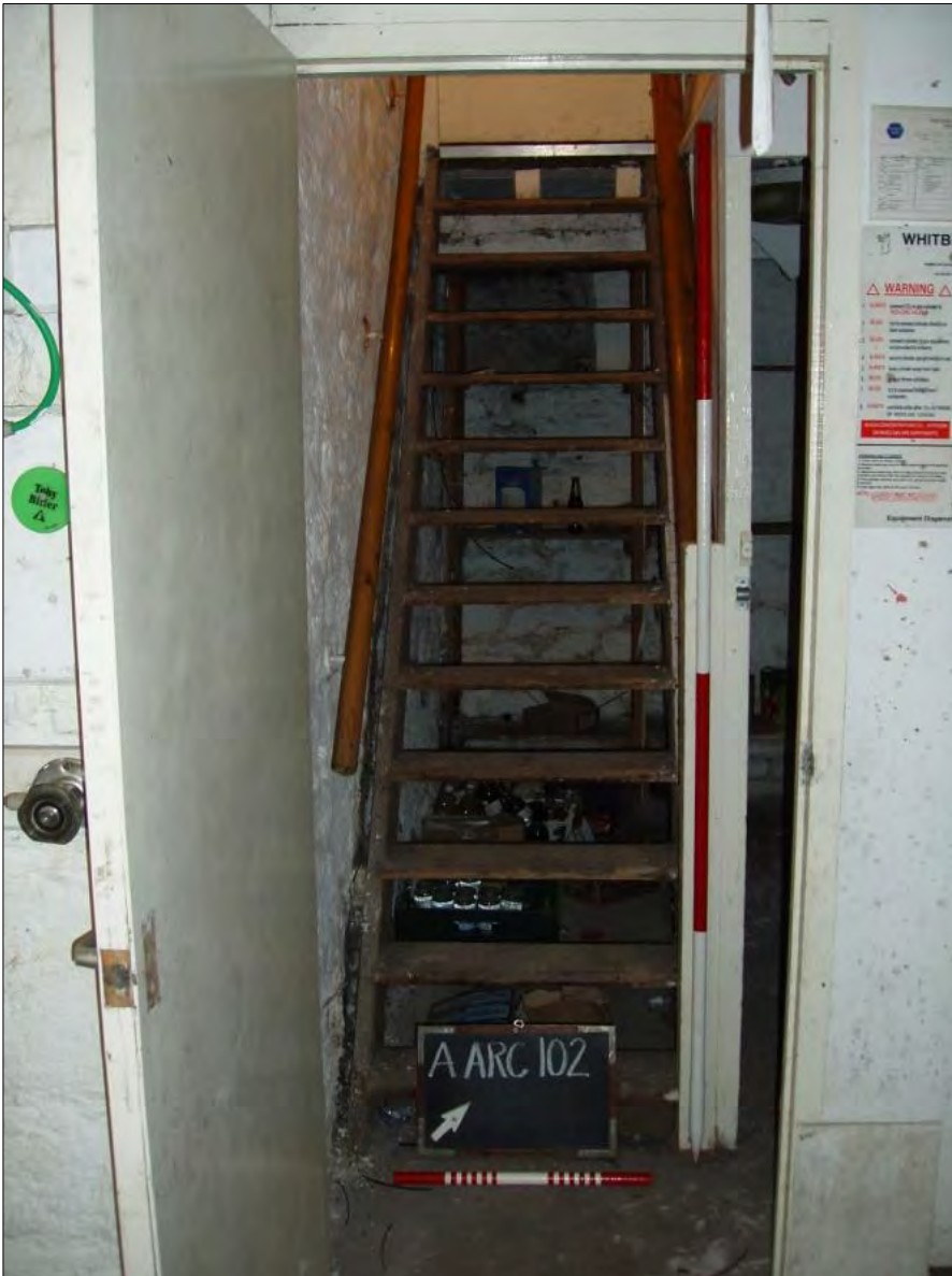
Photograph 8 NW View of Flight of Wooden Stairs- from Cellar to First Floor (Scales 1 x 2m & 1 x 500mm)
