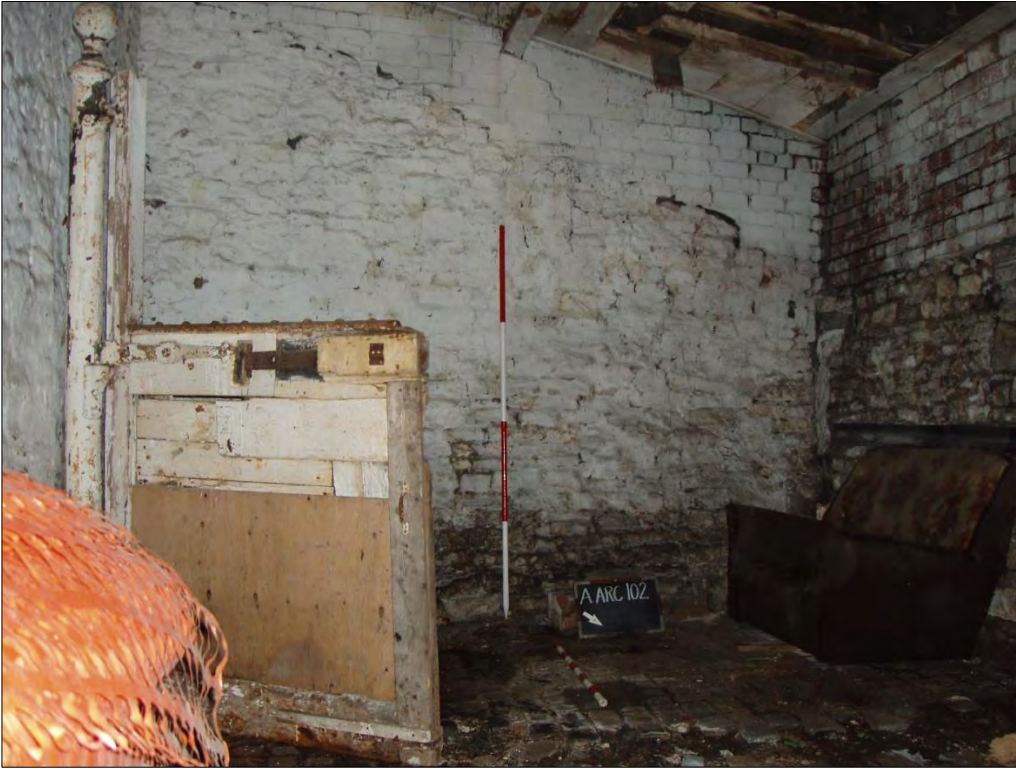
Photograph 37 West Facing View of Random Coursed Stone Wall with Brick Elevation to Raised Mono Pitch Roof to the Rear (Scales 1 x 2m & 1 x 1m)
