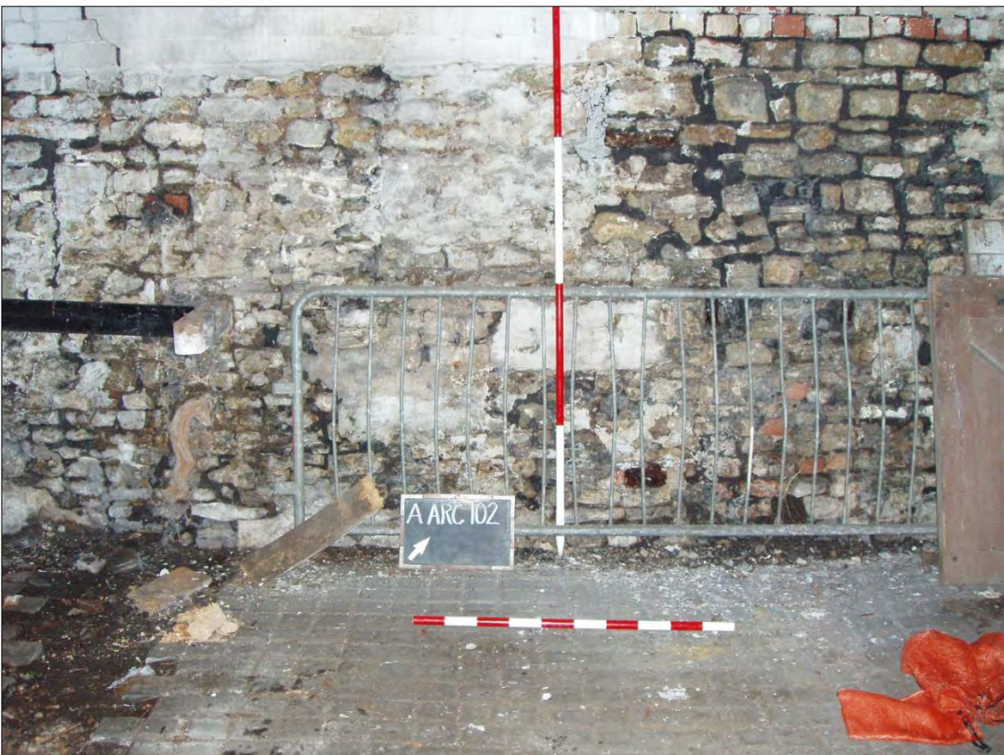
Photograph 38 NW Facing View of Random Coursed Rubble and Brick Wall (Scales 1 x 2m & 1 x 1m)
