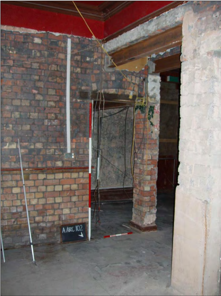
Photograph 14 Internal East Facing Elevation Showing Original Door Frame and Knocked Through Access in Foreground (Scales 1 x 2m & 1 x 500mm)
