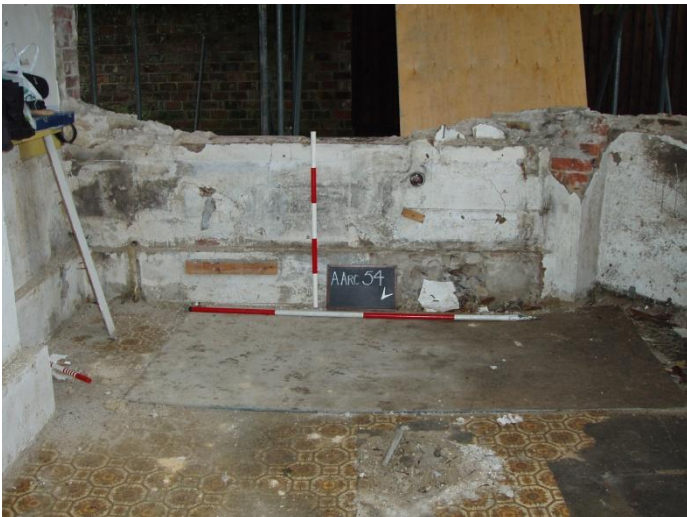
Photograph 3: SE Facing View of Extension Pre Demolition of Lower Coursing (Scales 1 x 1m & 1 x 2m)
