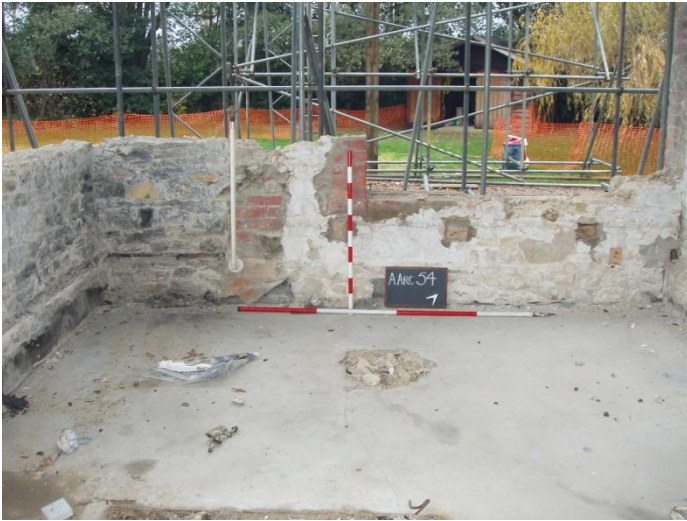
Photograph 1: NW Facing View of Extension Pre Demolition of Lower Coursing (Scales 1 x 1m & 1 x 2m)
