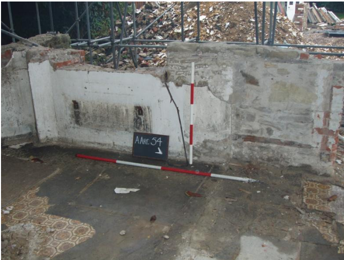
Photograph 2: SW Facing View of Extension Pre Demolition of Lower Coursing (Scales 1 x 1m & 1 x 2m)
