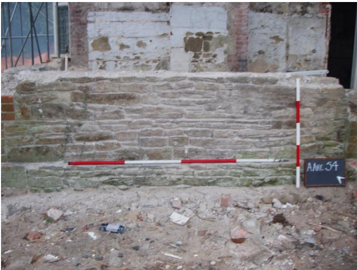
Photograph 4: NE Facing View of Extension Pre Demolition of Lower Coursing (Scales 1 x 1m & 1 x 2m)
