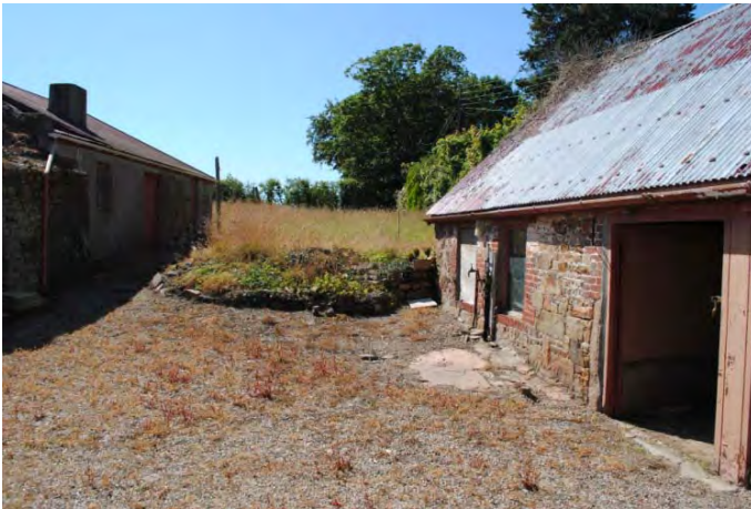
Photo 7: Area between Ruined Structure and Outbuilding, earmarked for levelling and extension of outbuilding (including the circular stone feature beneath the window) from E
