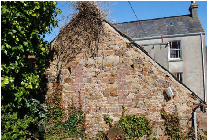
Photo 10: Gable end of outbuilding showing blocked window (2 nd floor) and alterations to the eaves
