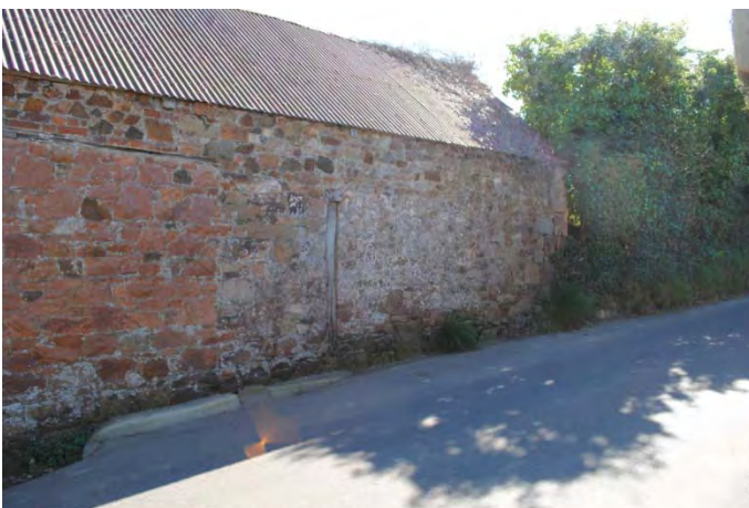
Photo 12: External view of western outbuilding from Le Rue du Ponterrin (N) showing post and joist also visible internally
