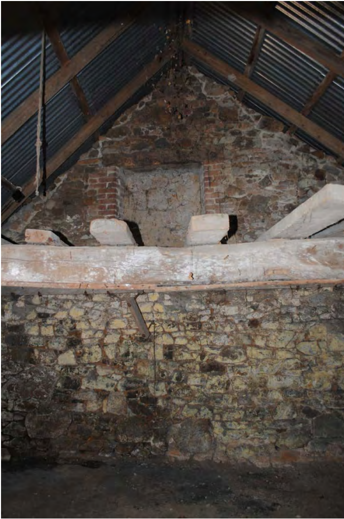
Photo 15: Internal view of west gable end of outbuilding with low joists and blocked up window
