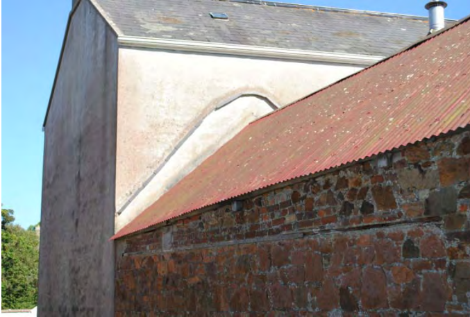
Photo 13: View of former roofline of previous building from La Rue du Ponterrin
