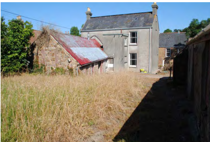
Photo 9: Ponterrin villa with 1950s flat roofed bathroom extension and outbuilding to W
