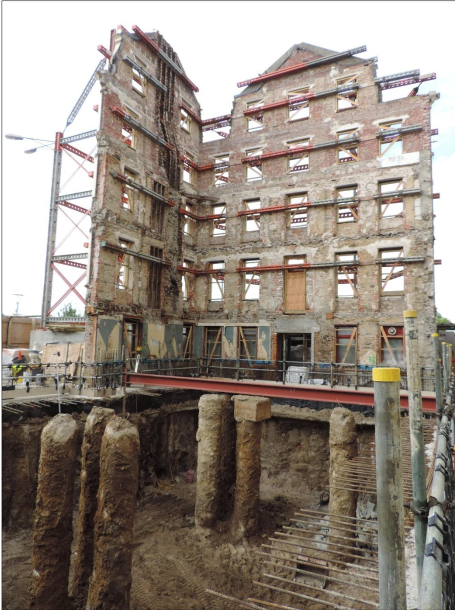
Figure 2 SW facing view of the Southamption Hotel façade during the ground reduction
