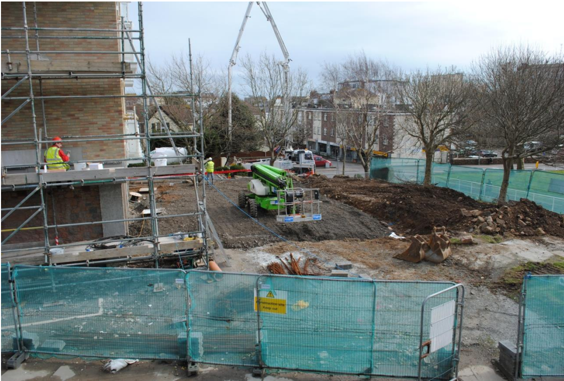
Photo 7: View looking east (and standing atop the raised grass area) of ground works associated with the high rise flat which were underway during site visit. A pile of rubble visible in the right of the picture included granite blocks.
