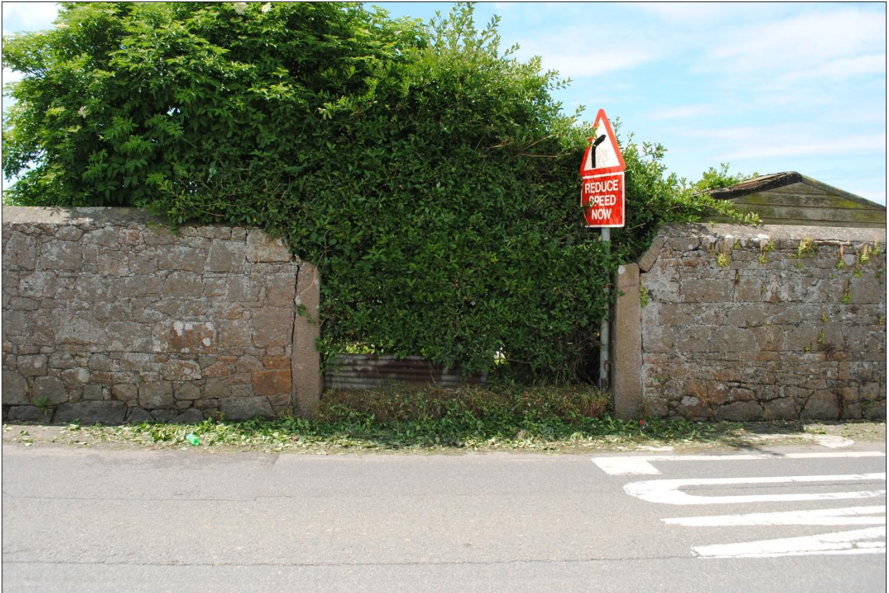
Photo 2 Granite wall and disused gate leading onto farm. SW facing view from La Rue Carrée.
