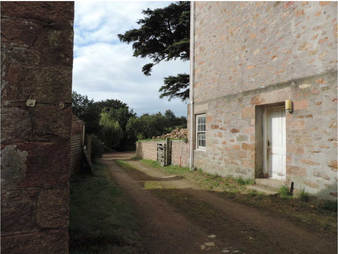
Photo 8: View of the east of Manor House, with door to basement (on right of image) and retaining wall in the background. This wall is not keyed in and was clearly added later
