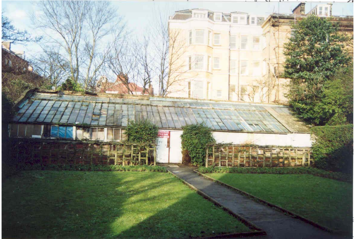
The rear garden in 1994 just prior to the demolition of the large lean-to greenhouse against the north retaining wall – this green house shown on the 1929, and 1939, 1:2500 scale OS maps and the 1965, 1:1250 scale map
