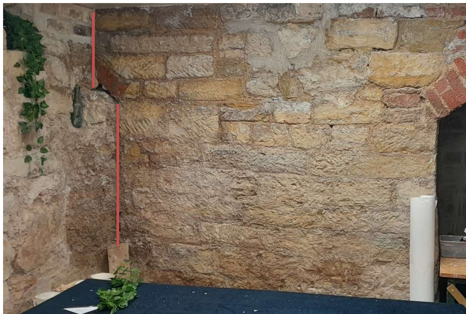
The west end of the north wall at its junction with the side wall showing the small section of visible brick arch abutted by the later side wall. Straight joints are indicated by the red lines
